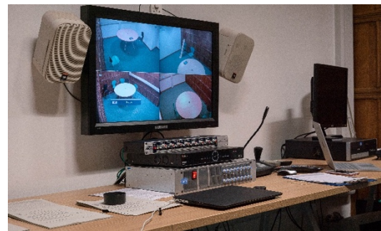
Observation Room equipment
