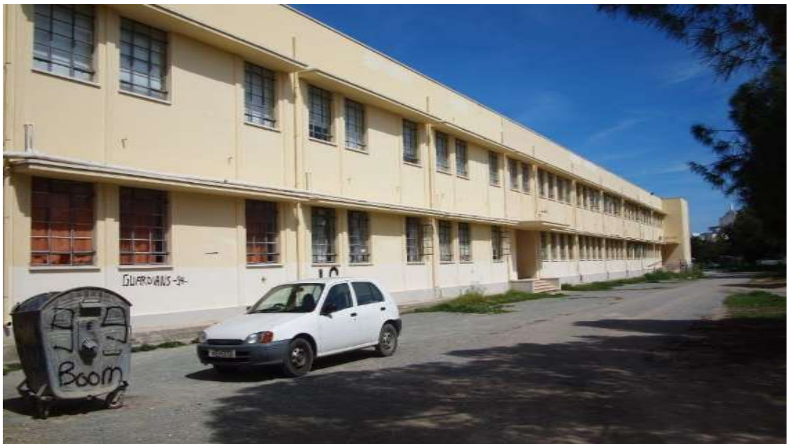
Il. 4- 20/ AGHS The south facade of the school, view towards the northeast @ Author, March 2018
