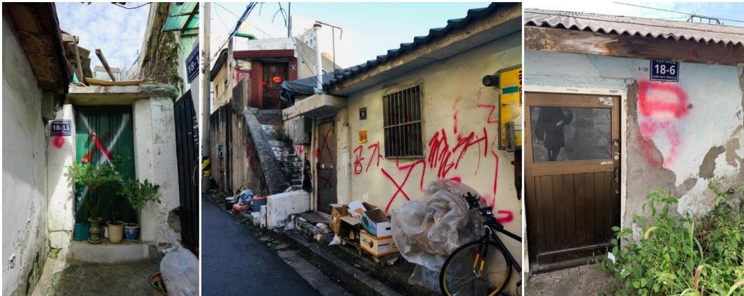
Figure 3-10. Spray-painted red markers on vacant houses in Nam-gu, Incheon
