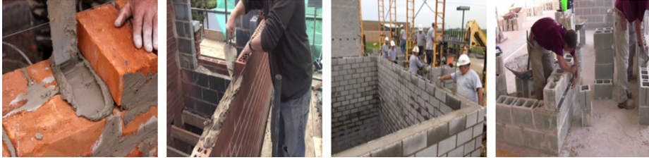
Figure 2-1. Examples of high intra-variability of masonry work with wide-ranging appearances and configuration
