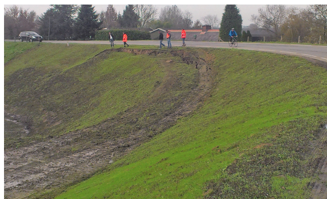
Figure 1: Slope instability without flooding.
