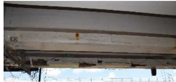
Figure 2: Damage on girders.
