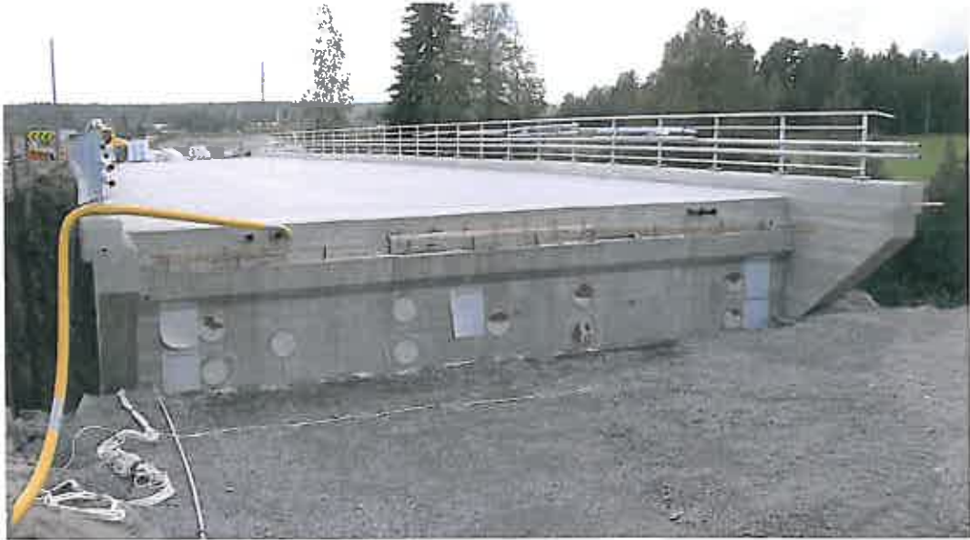
Figure 9.1.1. Instrumentation of the integral abutment bridge on Highway 9 in 2003.
