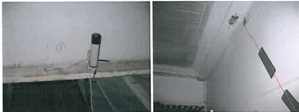
Figure 5.1.3. In the Hännilänsalmi bridge the strain gages have been fixed on the flanges of I-shaped beams.
