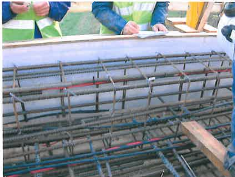
Figure 4.2.2. Installed Sahlen sensor (white device in the middle of the photo) close to the reinforcement.
