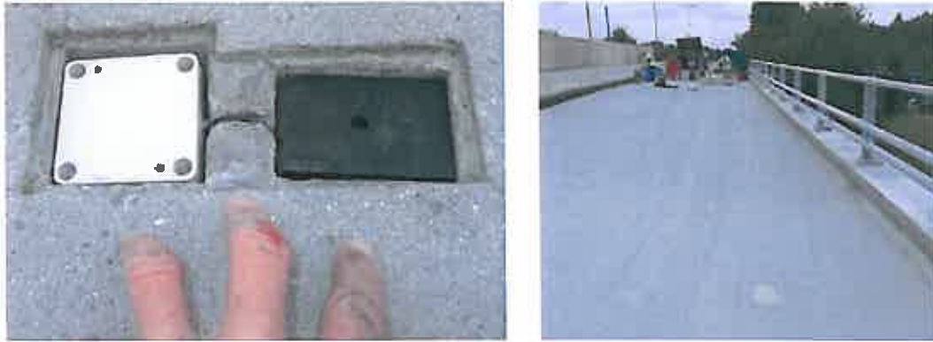
Figure 12.2.3. Battery pack on the left and the sensor on the right (left picture). The row of sensors is visible before installation of waterproofing membrane and asphalt (right picture). The battery pack and sensor are covered with 6mm thick teflon protection plate to protect them from open flames during the installation of the bituminous waterproofing membrane.
