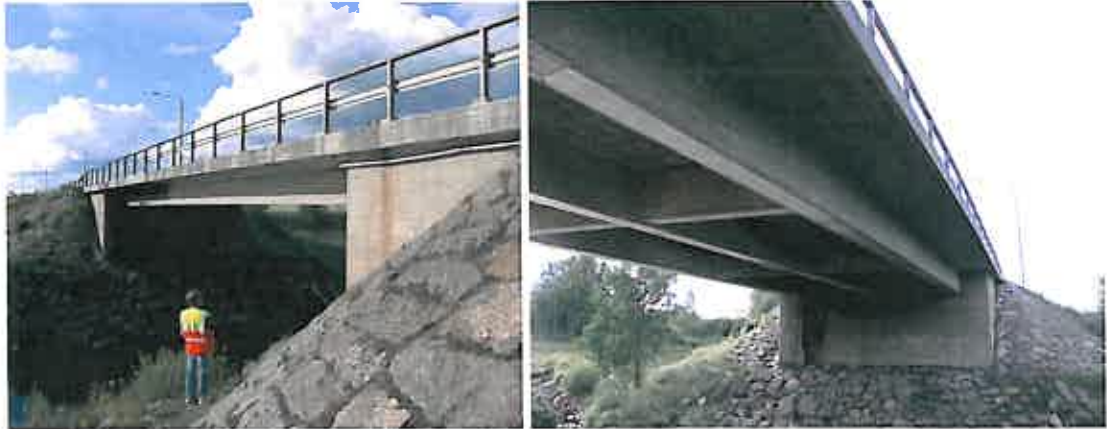
Figure 6.3.1. Jylhäranta Bridge. Glued steel plates under the main girders are shown in left picture.
