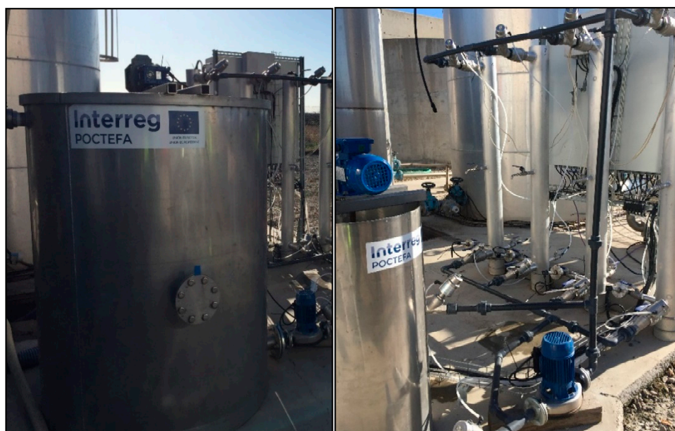
Figure 2. Pilot-scale plant process images.
