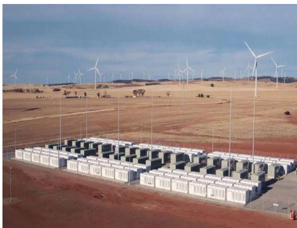
Fig.1. Large-scale battery storage system [12]
