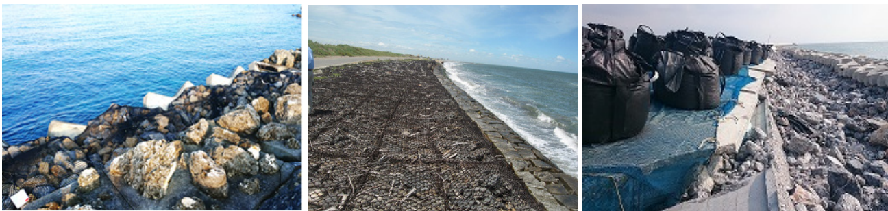
Fig. 1. Temporary armor units at the actual place (left: SFNs, center: Gabions, right: Sandbags ).
