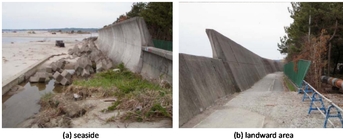
Fig. 1. Photograph of the cross-section changing dike in Nakoso District in Fukushima prefecture, Japan: (a) seaside view (b) landside view (NILIM (2011)).
