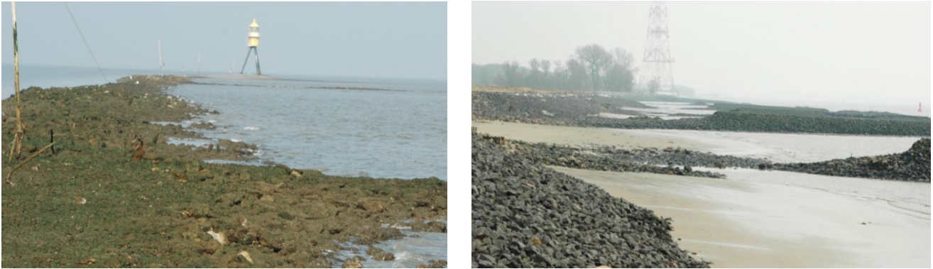
Fig. 1. Examples of ship-induced damage to rock structures: deterioration at training wall Langlütjen, Weser Estuary (left), damaged groyne roots at Juelssand, Elbe Estuary (right).
