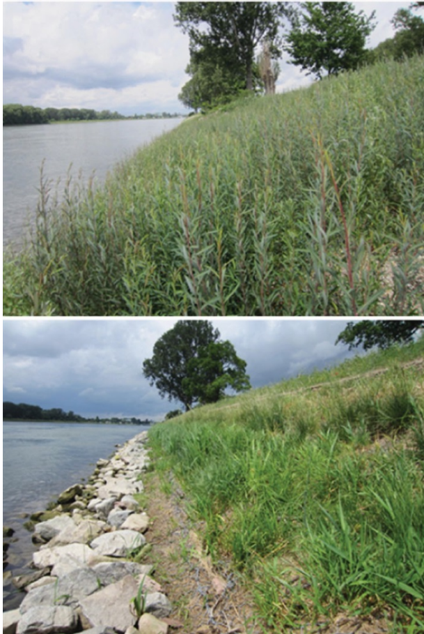
Figure 1. Two examples of technical-biological bank protections on the Rhine (upper picture: willow brush mattresses, lower picture: vegetated gabions, both 7 months after installation).
