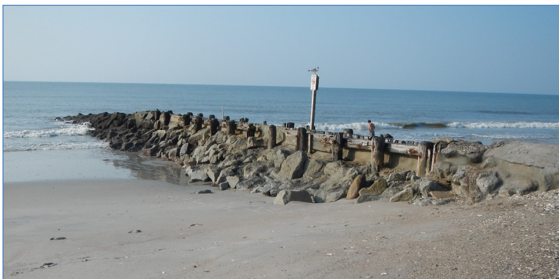
Fig. 4. Typical groin condition prior to the 2017 extension project.
