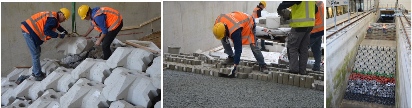
Fig. 7. Placement of Levvel-blocs (left), placement of Quattroblocks (middle) and finished structure of section 8 (right).
