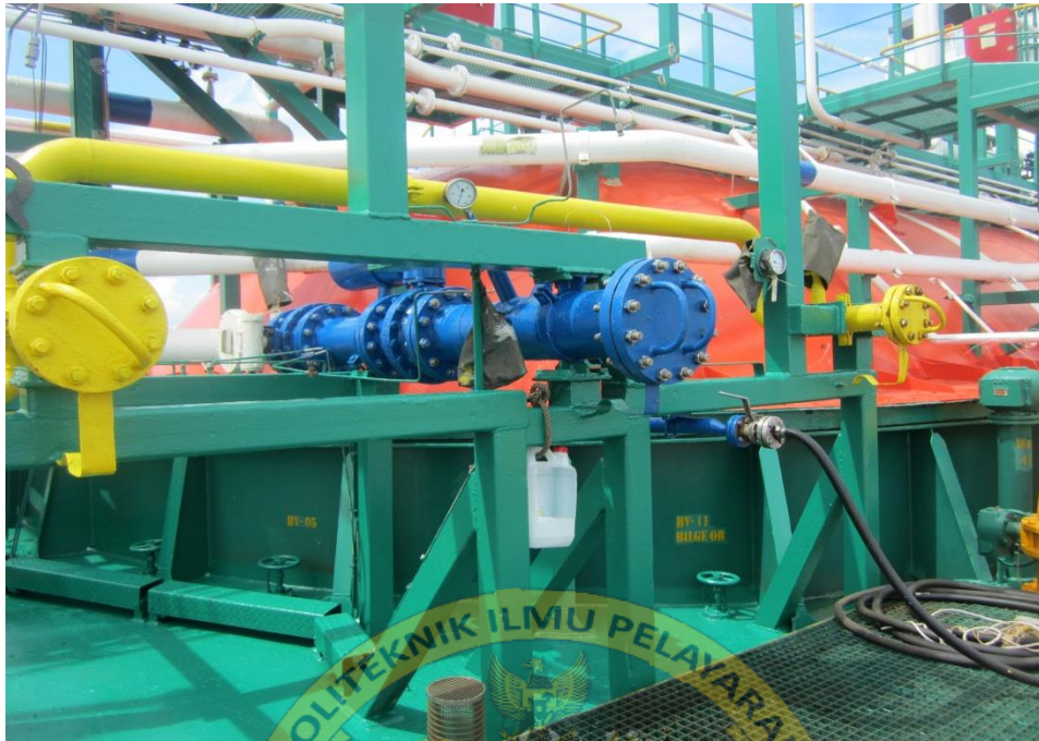
Gambar: Manifold LPG/C Gas Arjuna.
