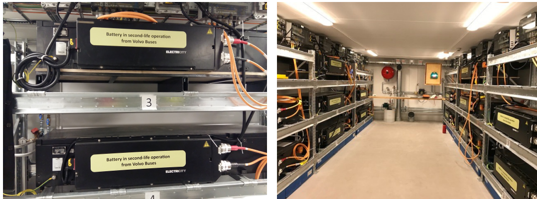
Figure 5.8: The second-life Li-ion batteries of Brf Viva.
