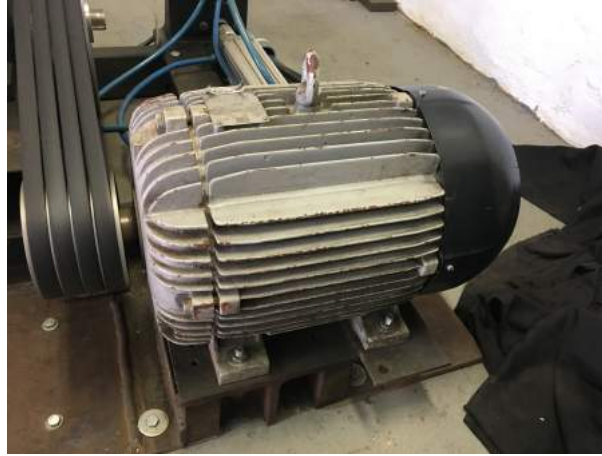
Figure 59 – Electric Motor WEG
