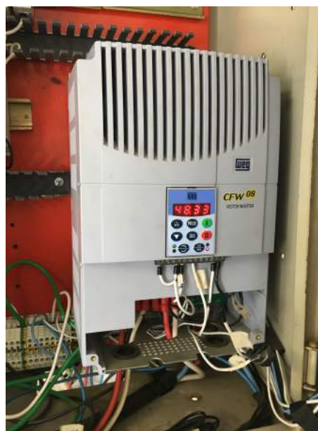
Figure 58 – Frequency Inverter WEG-CFW08
