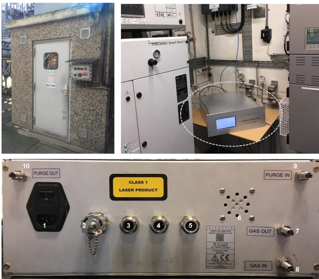
Figure 5. The sensor system in the analyzer house at Preem refinery (top images). The overview of connection ports on the rear panel (bottom image). The corresponding numbers refer to: (1) power inlet 230VAC 50Hz, (2) service ethernet port RJ-45, (3),(4),(5) I/O cable glands, (6) ventilation outlet, (7),(8) sample gas inlet/outlet, (9),(10) purge inlet/outlet.
