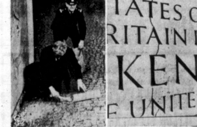
BOMB BLAST DAMAGES JFK MEMORIAL—Police brush away debris below a hole in the back of the Runnymede, England, memorial to the late President John F. Kennedy following a bomb blast which damaged the monument. The explosion opened a crack about an eighth of an inch wide all the way through the 7-ton block. (Cnblephoto)
