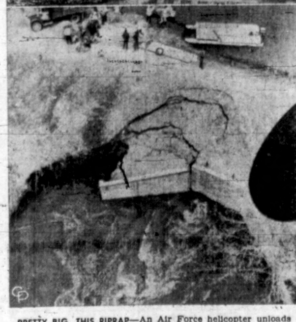
PRETTY BIG, THIS RIPRAP—An Air Force helicopter unloads an auto body into the Rock Creek levee break north of Quincy, Ill., which is being eaten away (lower) by the flooding Mississippi River. They also dropped old refrigerators.
