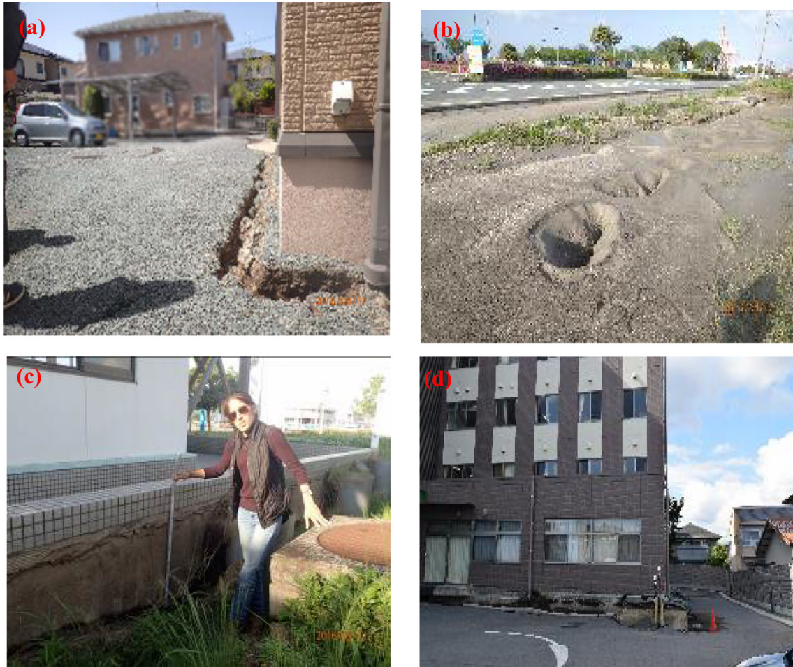
Fig. 2. Liquefaction-induced damage to buildings during 2016 Kumamoto earthquake: (a) Inclination of residential house, (b) Sand boiling and settlement, (c) Differential settlement of house, and (d) Settlement of building.
