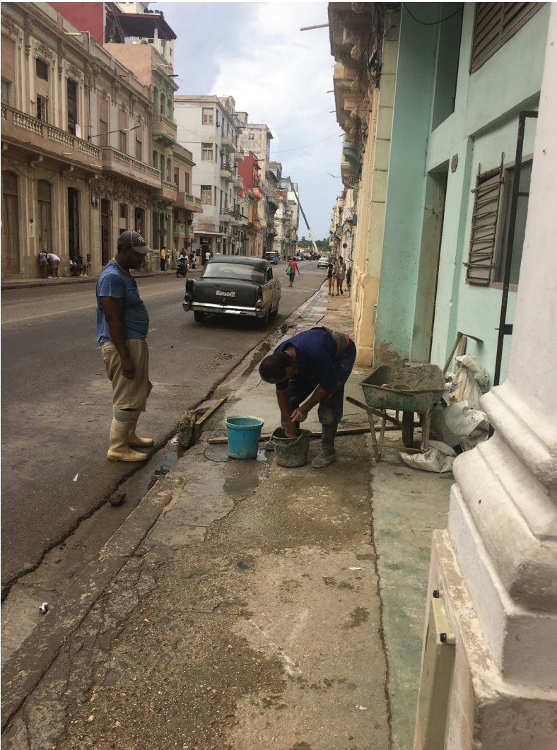
Figure 4. Two construction workers transforming a residential complex in Old Havana into a private hotel. Source: photo taken by Gertjan Wijburg
