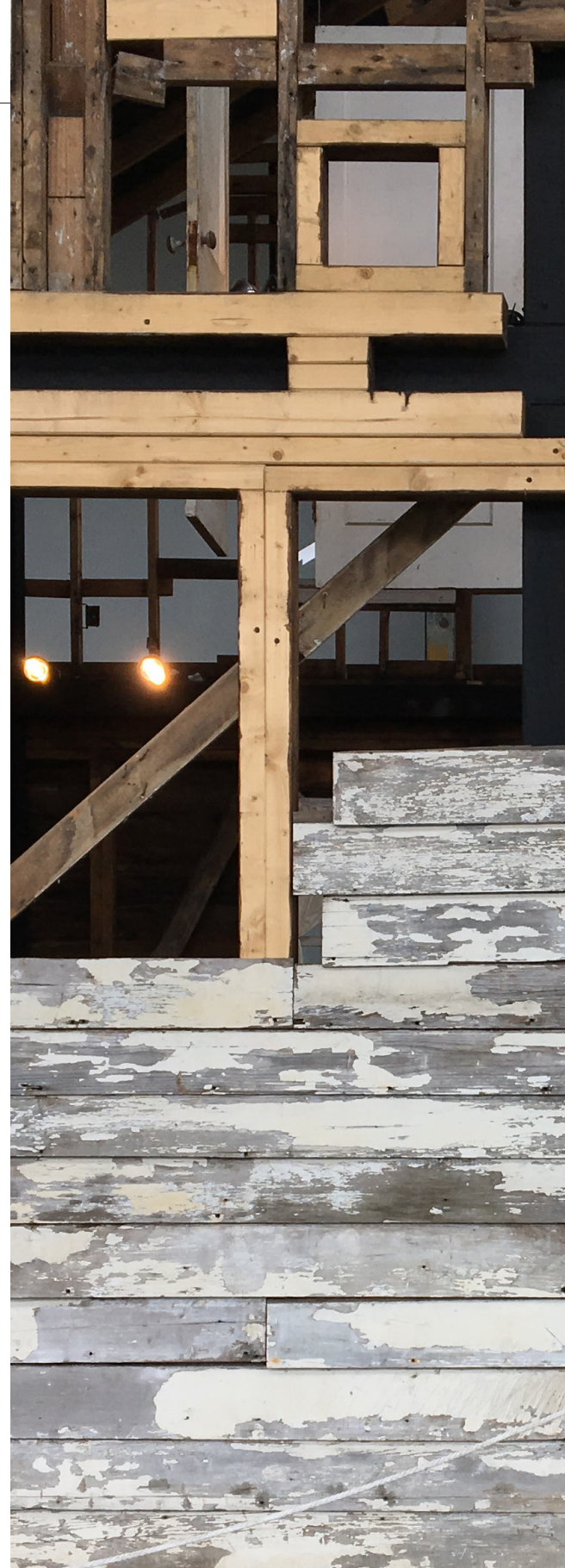
The side facade of 2672 S. Deacon Street in the process of reassembly at WaterFire Arts Center
