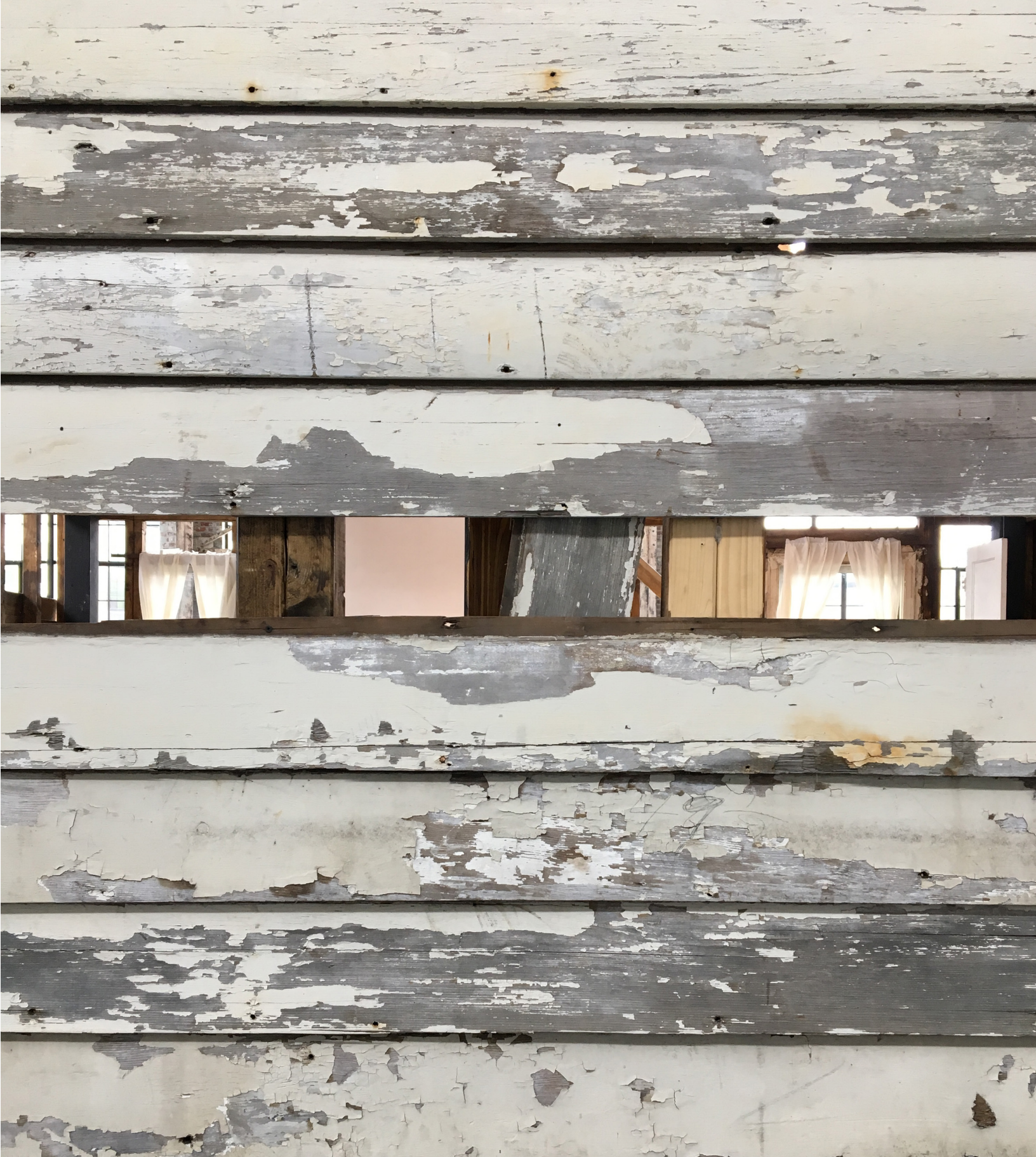
Closeup and through the clapboard to the interior of the Rosa Parks House Project
