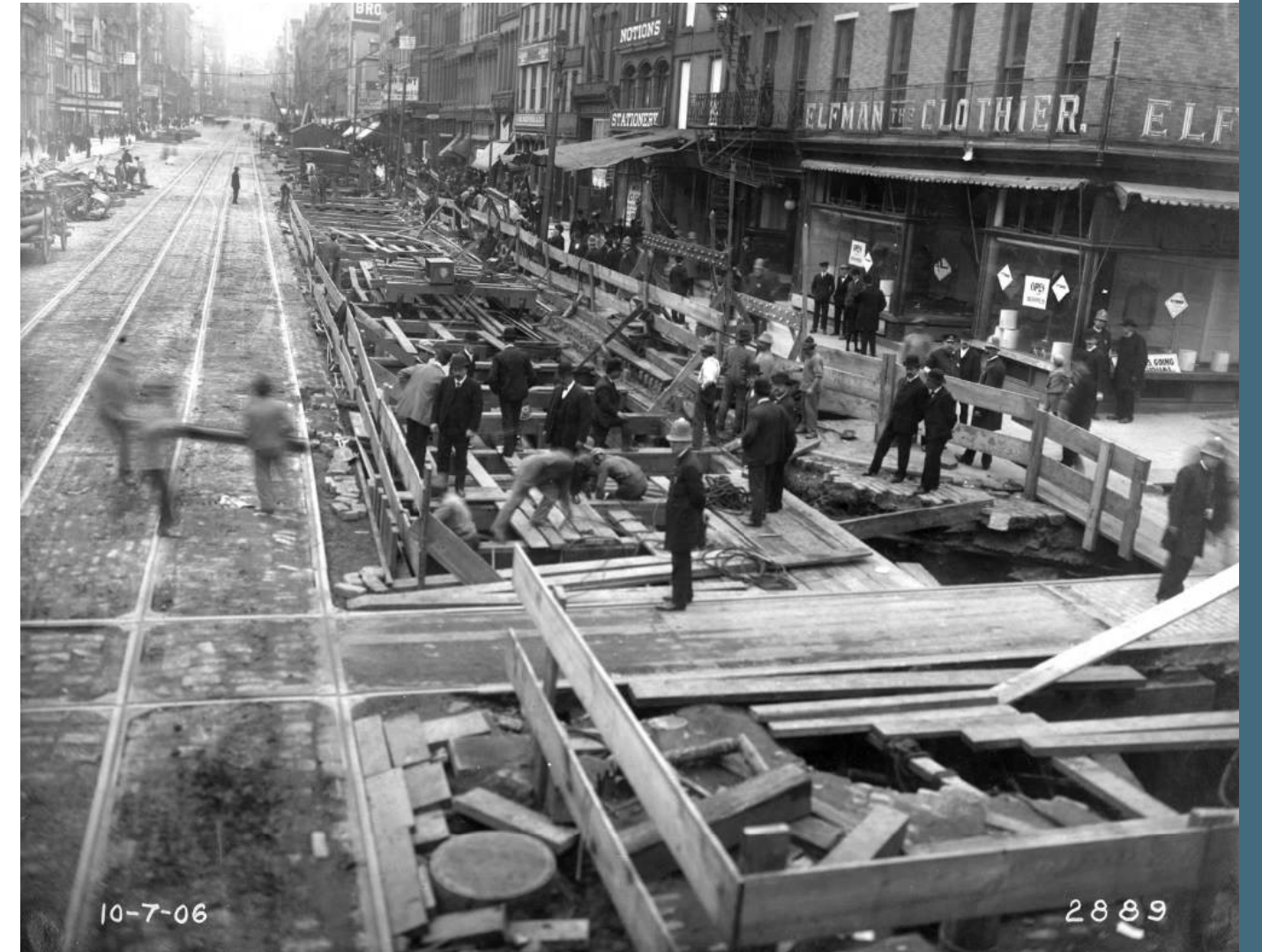
PHOTOGRAPH OF THE MARKET FRANKFORD LINE ELEVATED / SUBWAY TRAIN UNDER CONSTRUCTION ON MARKET STREET
