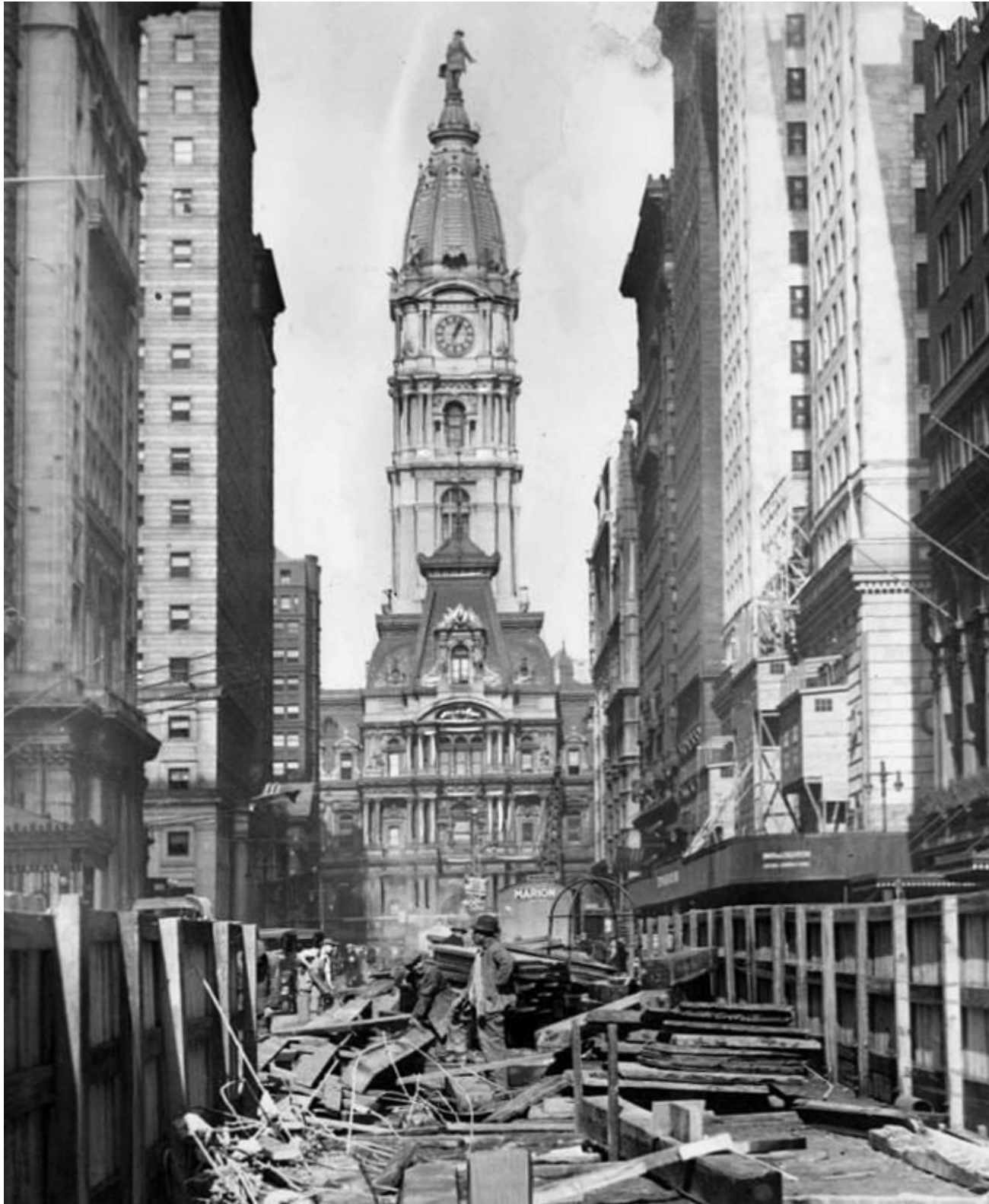
Construction of the Broad Street Subway line. Looking North on South Broad Street towards city hall, this image shows the excavation of the concourse level. This is part of a vast concourse system that exists today.
