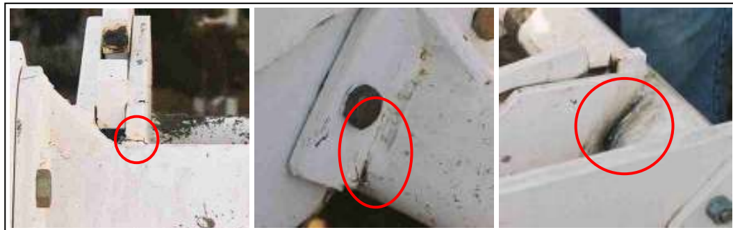
Figure 23: Cracks Found on the MCC
