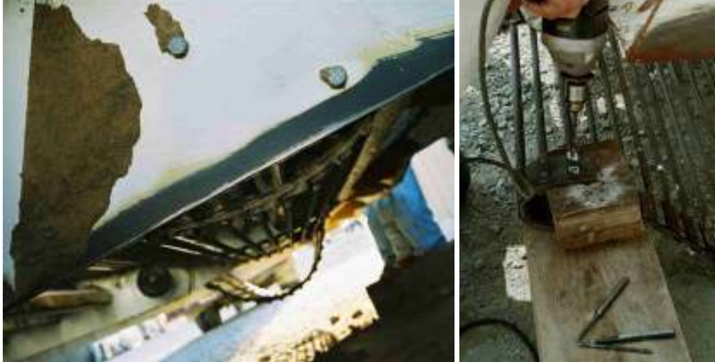
Figure 24: Loose MCS Belt Repair
