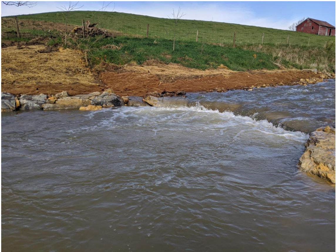
Figure 23. Implemented cross vane structure looking upstream Photo by Dylan Cooper, Trout Unlimited
