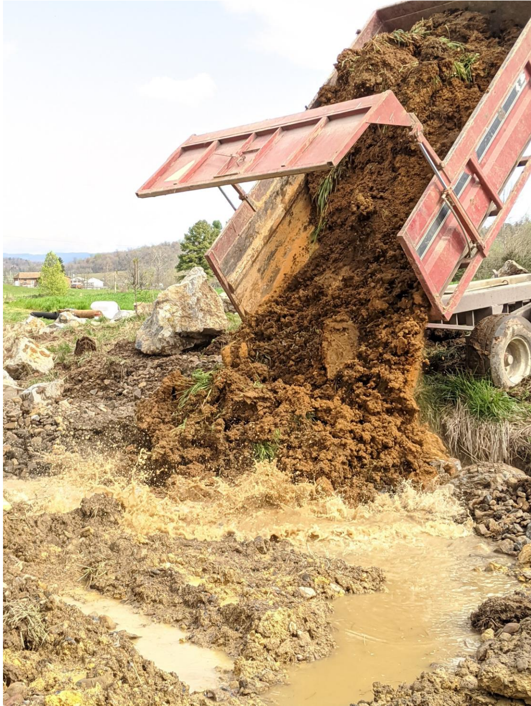
Figure 22. Sediment from excavated bar to fill eroded banks Photo by Dylan Cooper, Massanutten Chapter of Trout Unlimited
