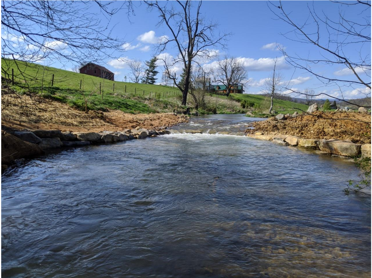
Figure G.1 Former bar location (looking upstream) that was excavated Photo by Dylan Cooper, Massanutten Chapter of Trout Unlimited
