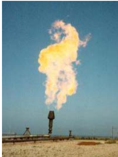
Figure 8: An Operating Coanda Flare
