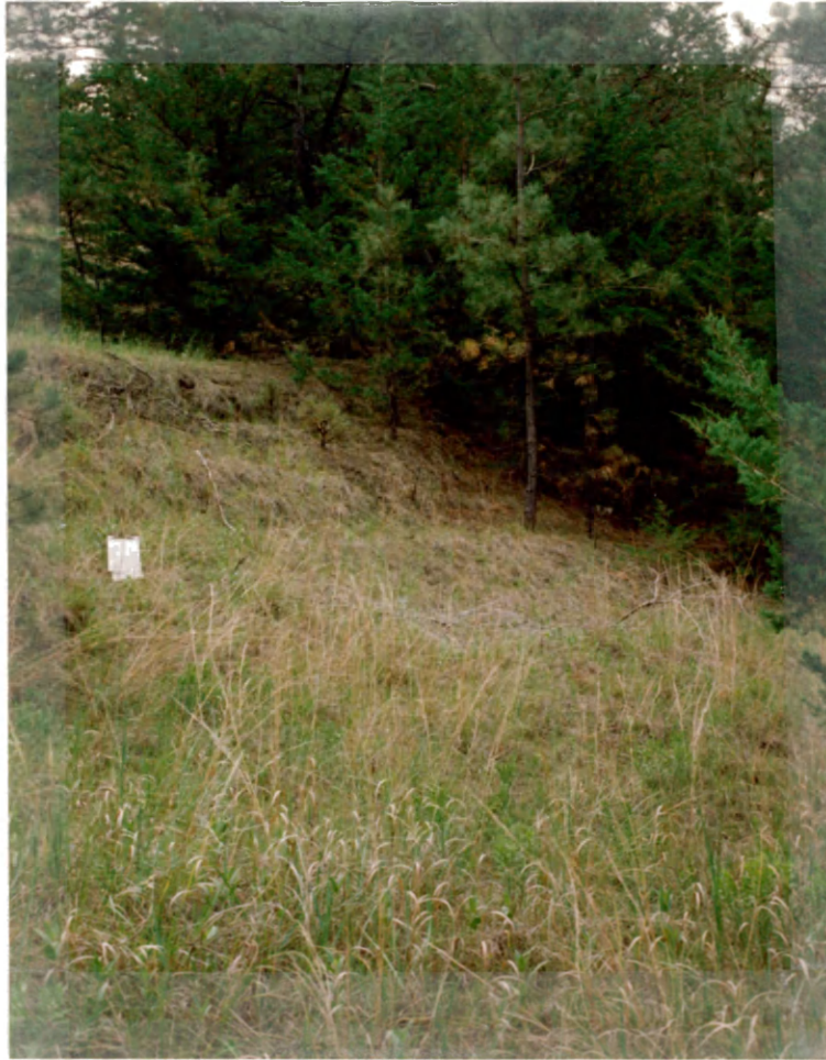
Fig. 33. Note the "steps in slope," an indication of slope failure. The size of the steps is one to one and half meter (photograph 1989).
