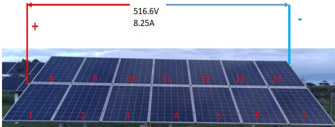
Figure 3. 3: A 3.5 kW module string at Outdoor Research Facility at Nelson Mandela University, string Voltage 516.6 V and current of 8.25 A.
