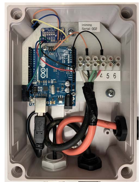
FIGURE 3. Assembly of the precision analog-to-serial converter (PASC) in a water-proof enclosure rated IP66.
