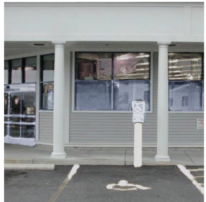
Details are critical to maintain long-term value. Plastic columns in this example are susceptible to snowplow damage. Bases are not flush with the pavement.
