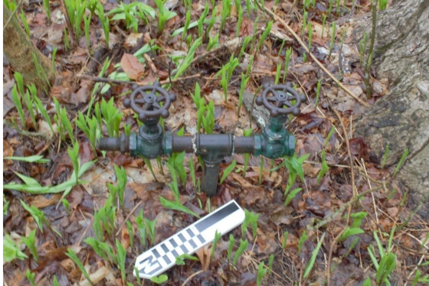
Figure 6.33: Photo of a T-shaped water valve.
