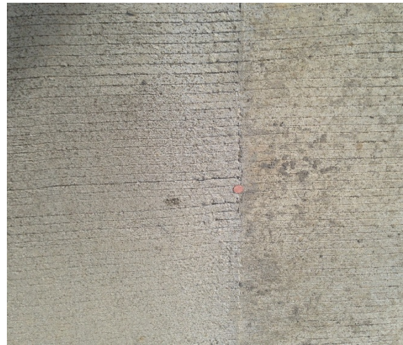
Figure 21 Cold joint at tie pour is partially exposed and partially covered with concrete slobber
