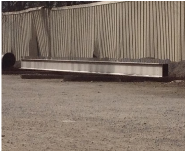
Figure 4 Inconsistent surface preparation
