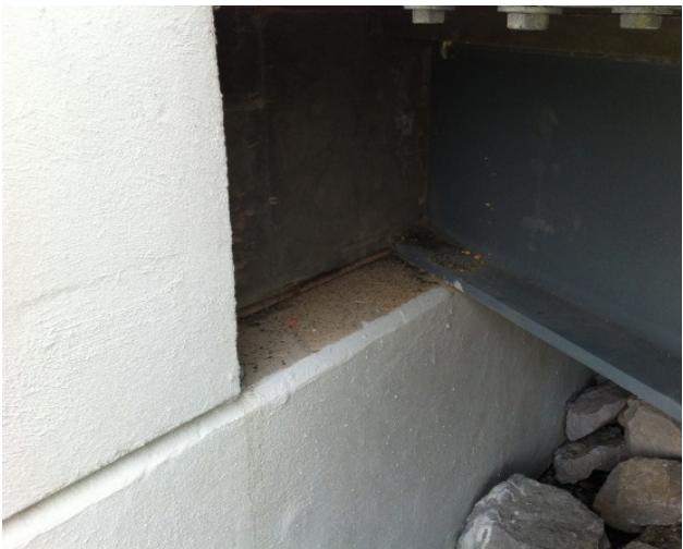
Figure 24 Concrete stain not applied on bearing area of abutment
