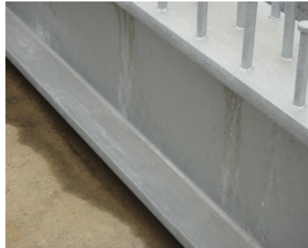
Figure 5 Inconsistent surface preparation reflected in the galvanizing
