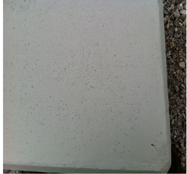
Figure 23 Concrete stain on bridge wing wall
