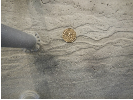
Figure 1 Top of Top Flange
