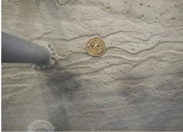
Figure 6 Thick – irregular galvanizing
