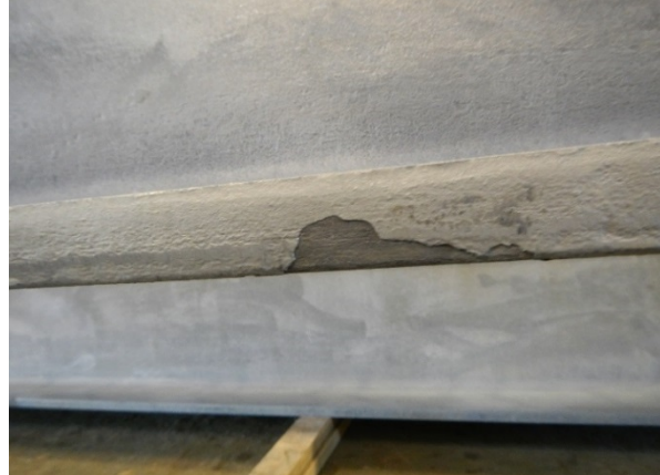
Figure 7 Cracks in galvanizing on the bottom flange
