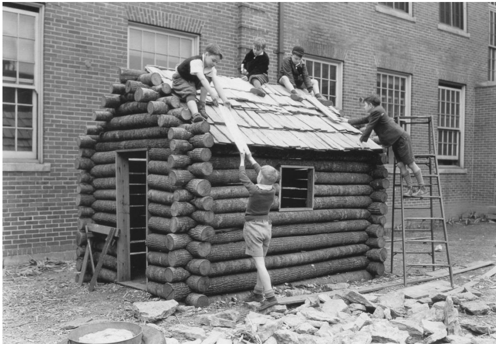
Figure 4.52: UK Teacher Training School: Students build a log cabin (University of Kentucky Archive)
