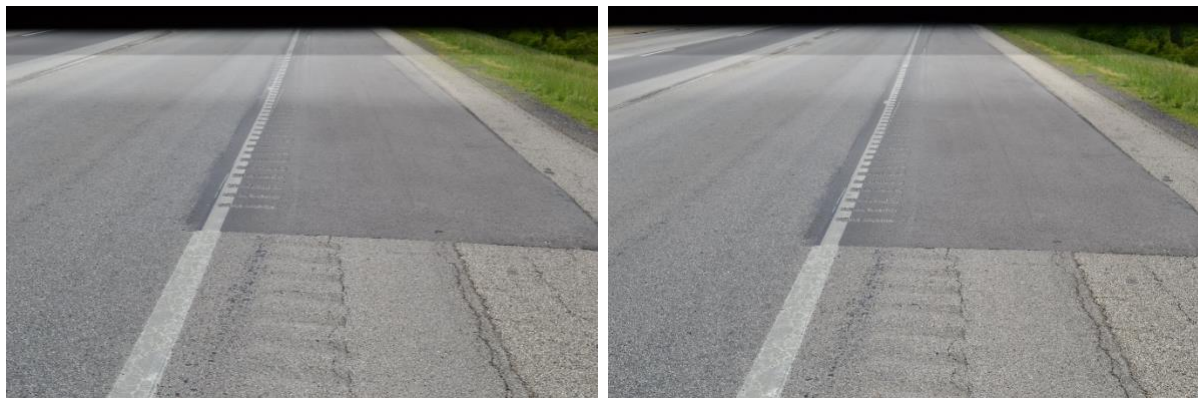
Figure 5.7 I-75 Shoulder Patch and Shifted Rumble Strip
