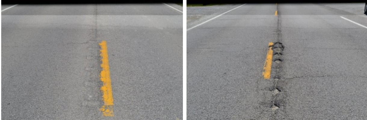
Figure 5.14 US-27 Centerline Rumble Strip Failure Due to Pavement Age
