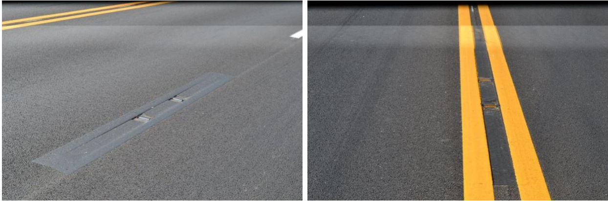
Figure 5.19 KY-80 Sealed Recessed Marker Pavement Grooves
