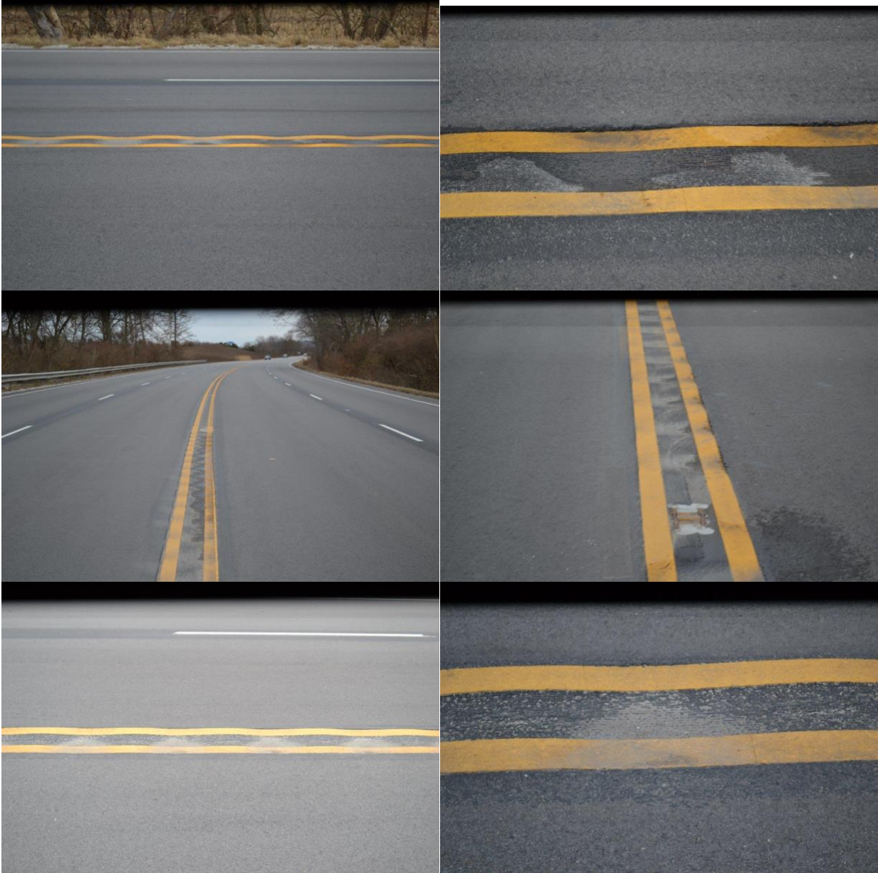
Figure 5.23 SR-50 Indiana Sinusoidal Centerline Rumble Strip
