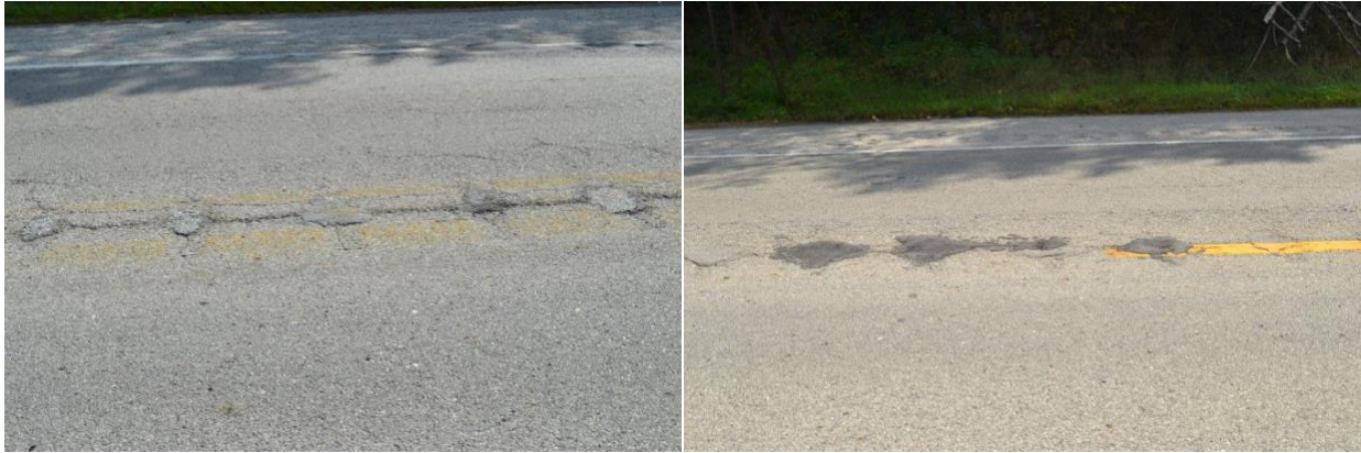
Figure 5.10 Mountain Parkway Centerline Rumble Strip Failure at Pavement Joint
