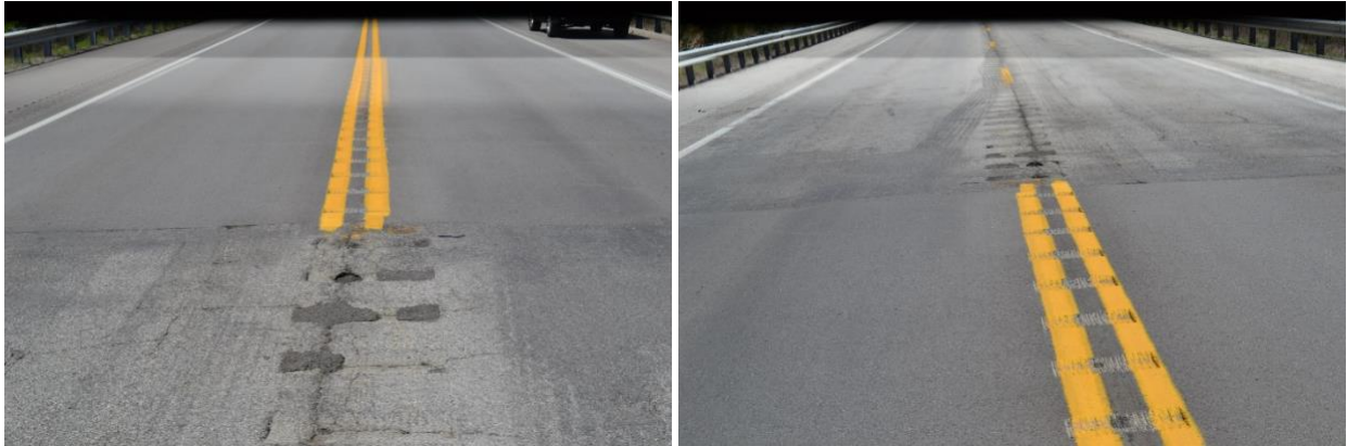
Figure 5.21 AA Highway Centerline Rumble Strip Durability Issues
