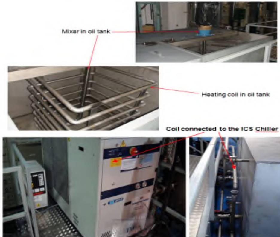
Figure 3-8: The 3-inch test facility chiller unit
