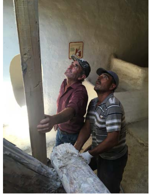
Figure 4: Ahmet Bülüç and Zekeriya Sivaz fixing roof of a model house (Photo by Berkay Dinçer).
