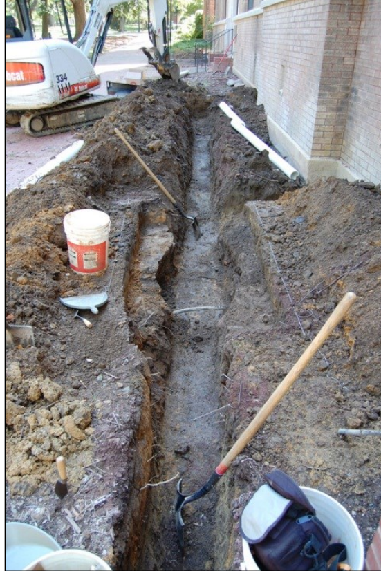
Figure 2. Preliminary archaeological investigation of the Vance site within the trench dug for drainage pipe installation.
