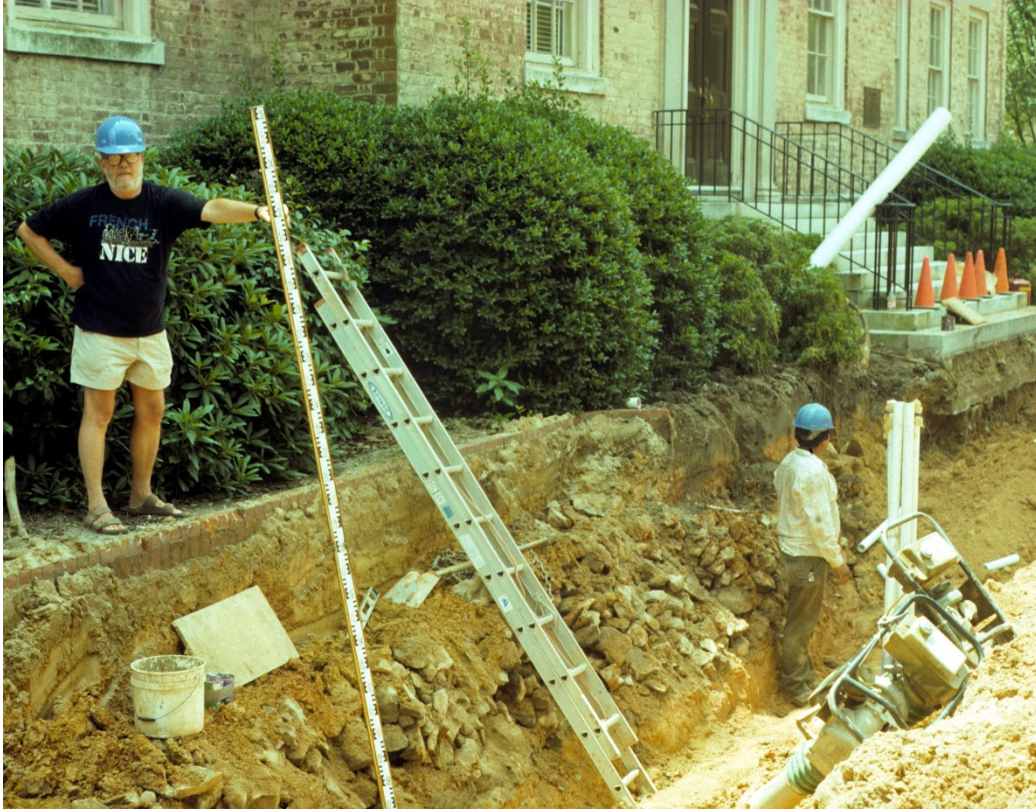
Figure 9. RLA archaeologist Trawick Ward standing above the stone drain uncovered in front of South Building in 1992.
