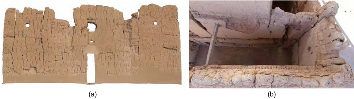
Fig. 5. (a) West perimeter wall showing large vertical cracks that appear opposite interior partitions and divide façade into several segments. Lens-shaped spalls near base of second wall segment may have occurred in an earthquake (Orthorectified image, Western Mapping Inc.); and (b) North perimeter wall showing extensive axial cracks (parallel to wall surfaces).
