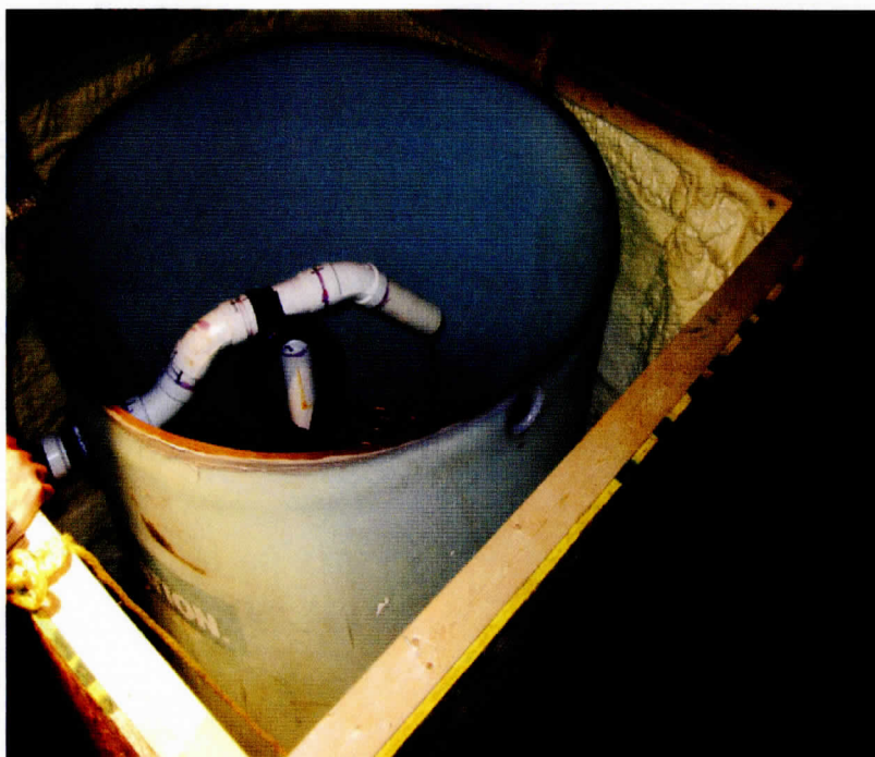
Figure 12. Tank enclosed in wooden box with closed cell spray foam insulation.
