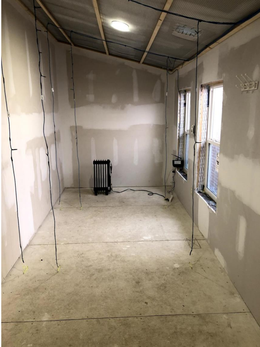
Figure 4. Temperature sensor network and radiant heater.
