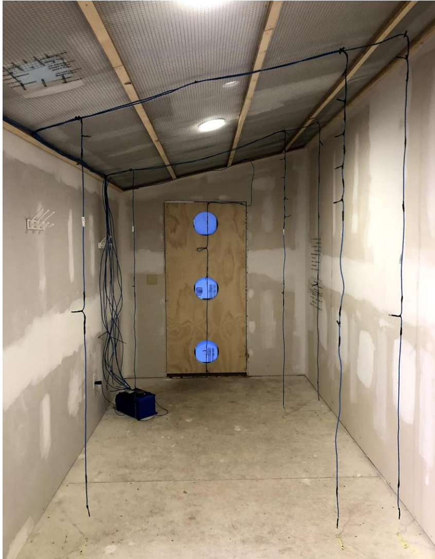
Figure 5. Temperature sensor network and custom blower door.
