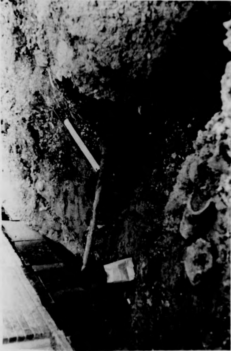
Figure 25. Waterproofing of West Wall and Replacement of Water Main Piping on the Exterior
