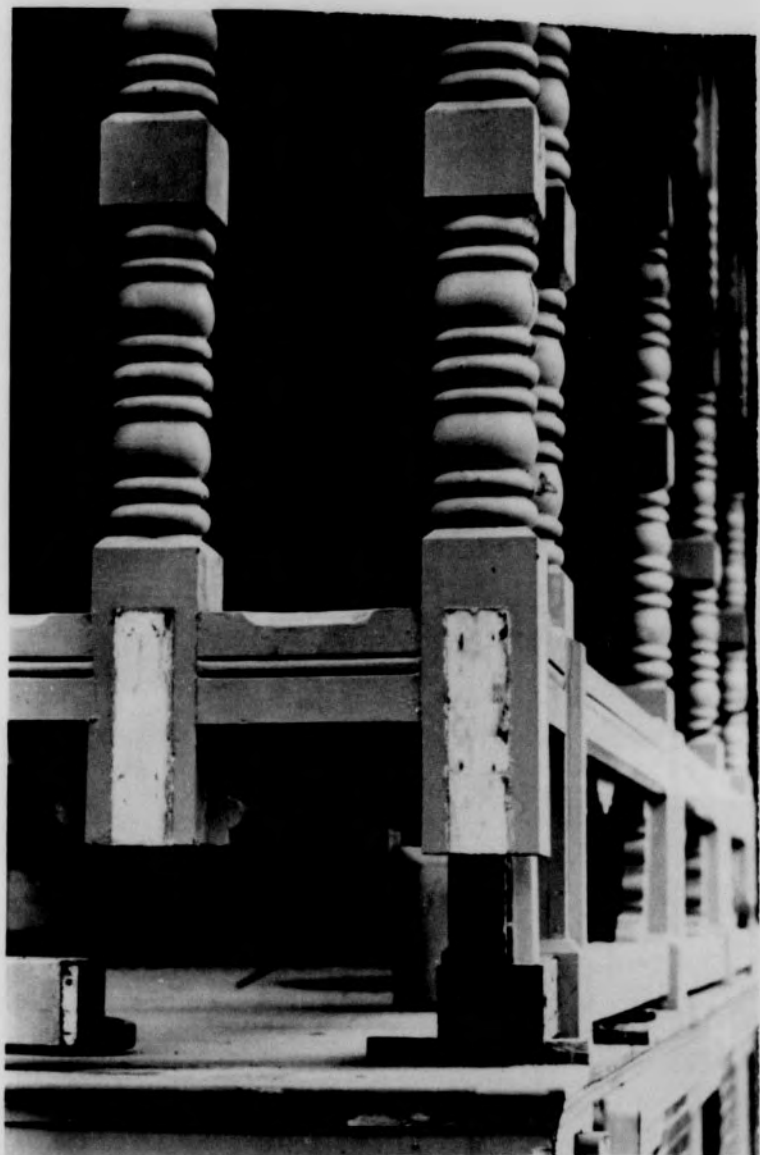
Figure 9. Rotten Wood Cut Out of a Column
