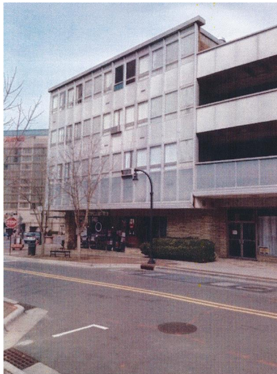
Figure 59. Street Façade Condition at the Beginning of the Project. (Hills, 2016)
