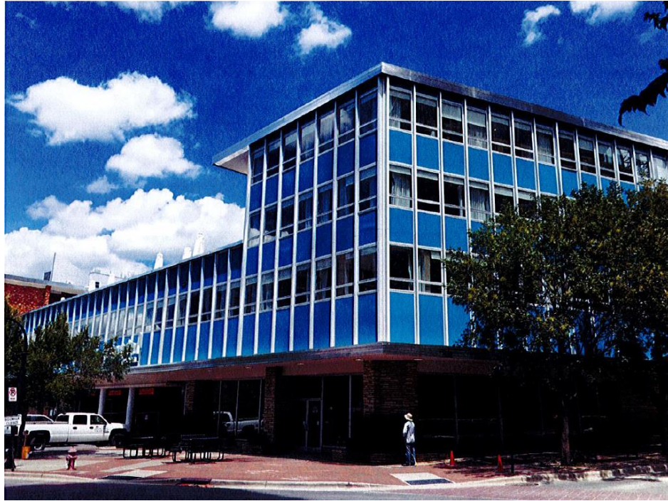
Figure 60. Curtain Wall on the Southwest Corner of the Building After Rehabilitation. (Hills, 2016).
