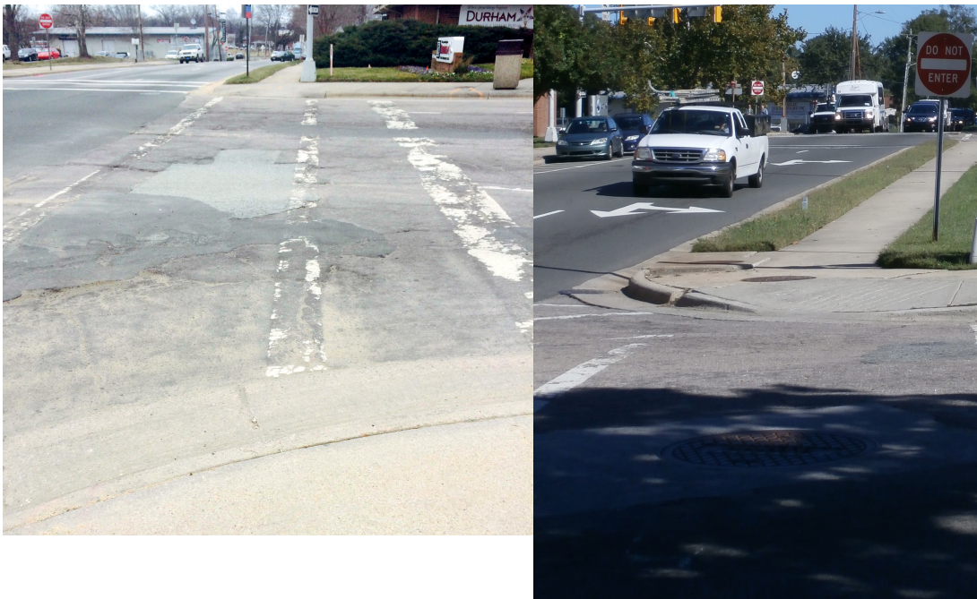
Figure 23. Photographs of PLOS Section 1. The left photograph shows the deteriorated condition of the crosswalk at the corner of W. Morgan Street and N. Mangum Street. The right photograph shows the sidewalk section used to calculate the worst PLOS score.
