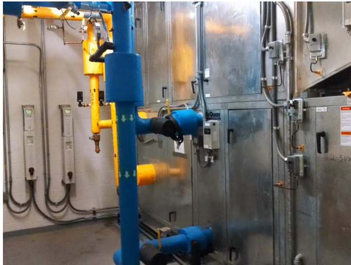
Air Handling Unit located in a Summit basement mechanical room.
