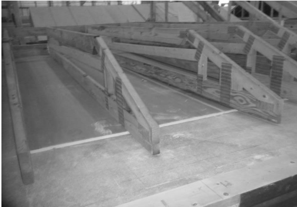
Figure 8. Knock-down, hinged trusses allow the sloped roofs of modular buildings to tilt-up on site, and transport flat (photo by author).
