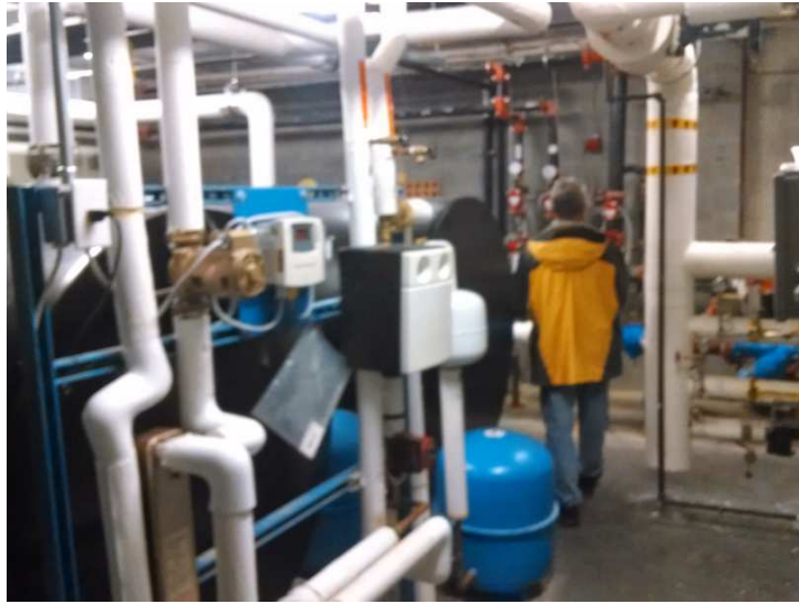
Mechanical room in Mountaineer with the solar thermal water heating balance of system shown.
