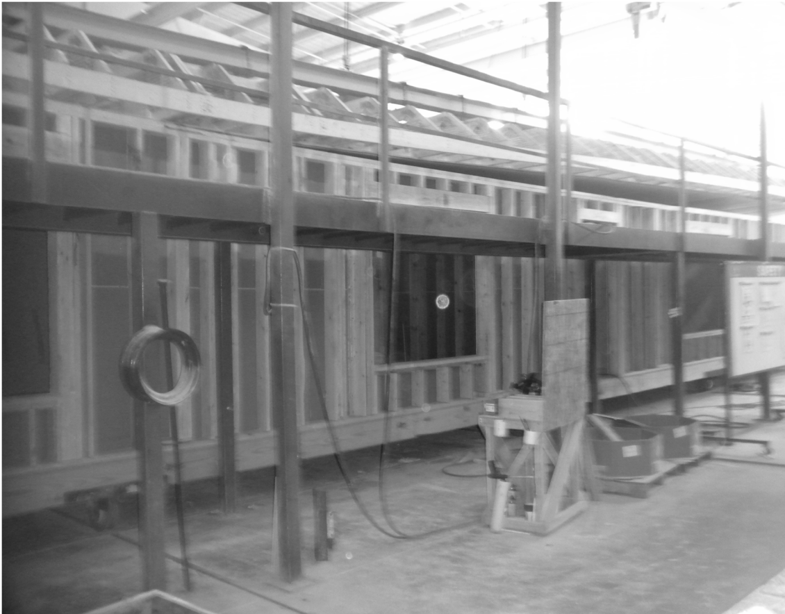
Figure 14. Permanent scaffolding erected around building modules on a factory floor (photo by author).
