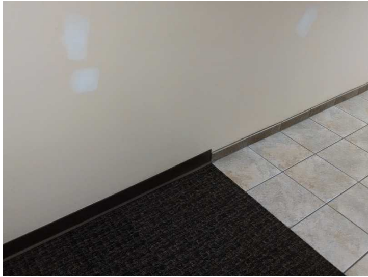
The transition between site-built work and a module is obvious at this juncture in the floor. It is barely perceptible in the picture, but under foot, the feeling between tile and carpet is distinct.
