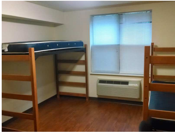
Typical dorm room in Mountaineer. Notice the PTAC unit located under the window, the wood-pattern vinyl flooring, and the chase in the upper left corner that routes the bath vent to the outside.
