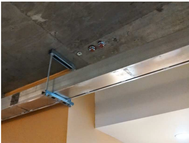
Exposed mechanical systems in Summit. Notice the two round penetrations filled with fire sealant. These were obviously misplaced, illustrating the difficulty of making changes in concrete buildings.
