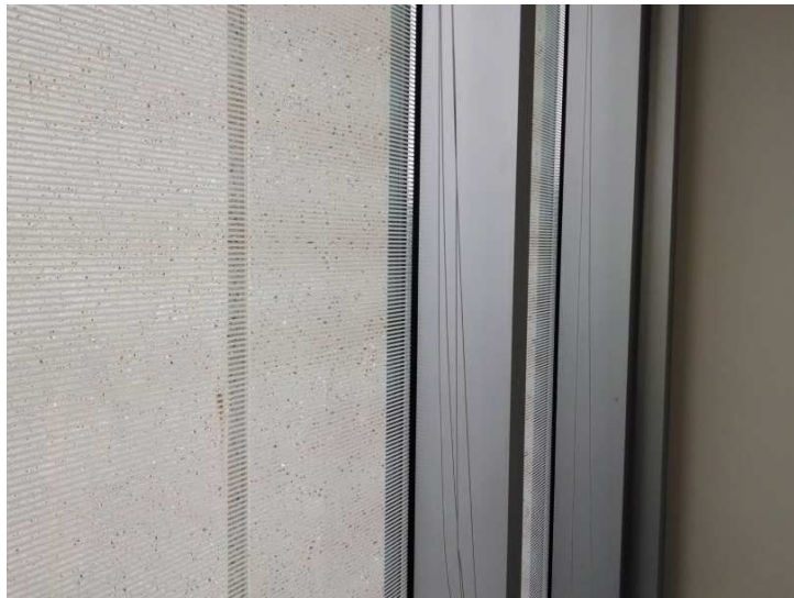
Fritted glass on the south walls of Summit that is intended to regulate solar heat gain.
