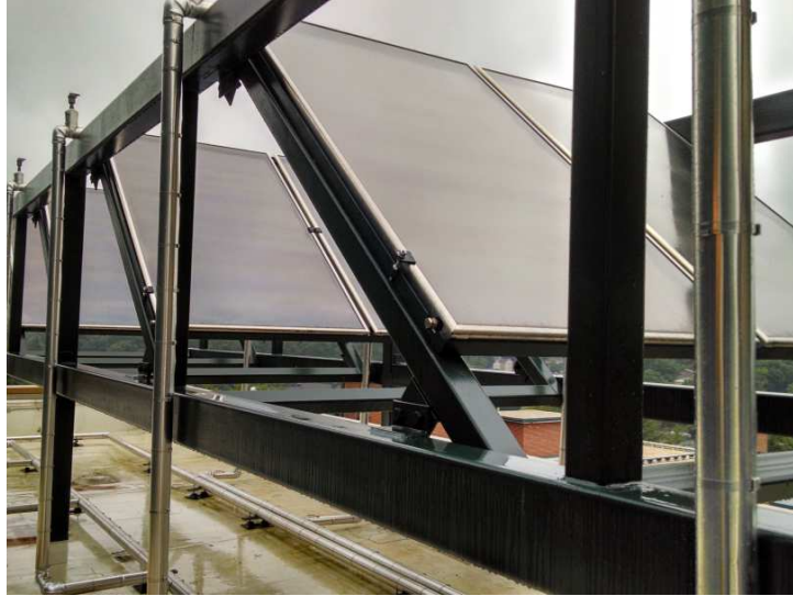
Solar thermal collectors and racking on the roof of Summit.
