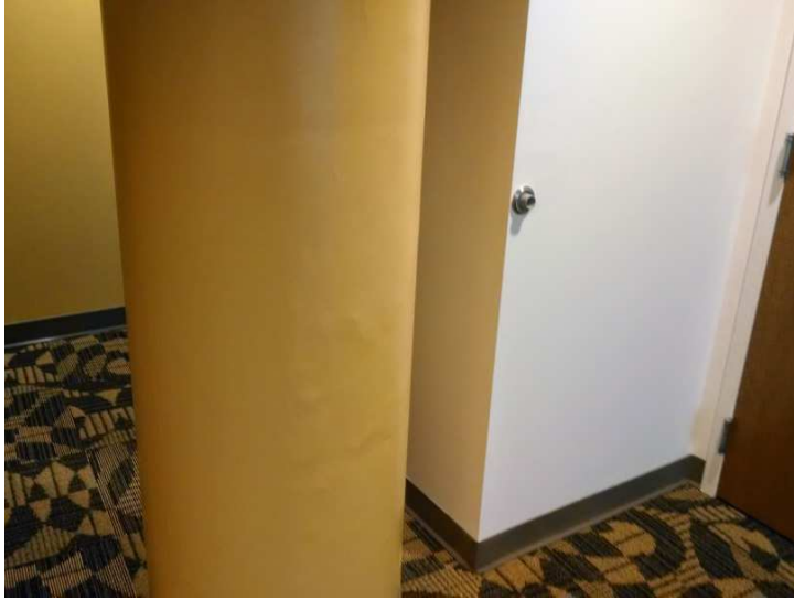
Similar to Mountaineer, there are elements in Summit that are not the highest quality such as the concrete finish on this column.
