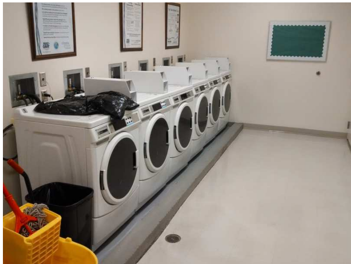
Laundry facility in Summit that is similar to that of Mountaineer.
