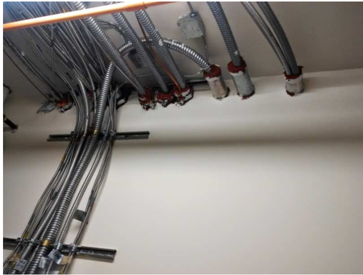
All electrical wires are Metal Clad (MC) cables at Mountaineer.
