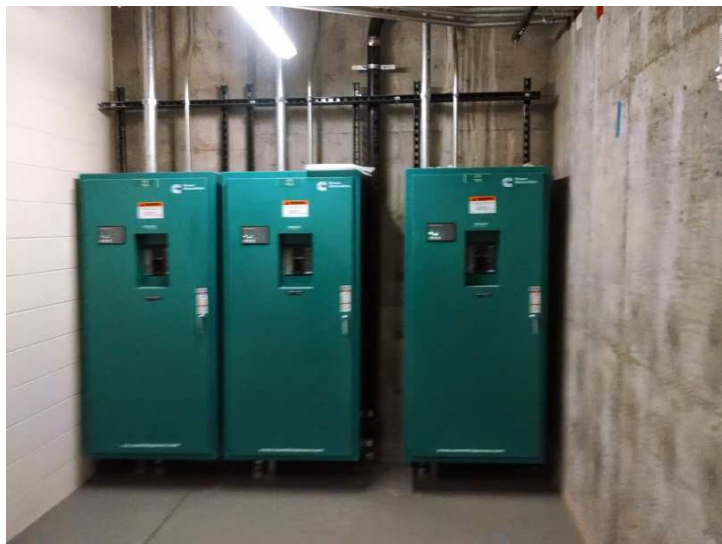
Interior electrical components of Summit generator.
