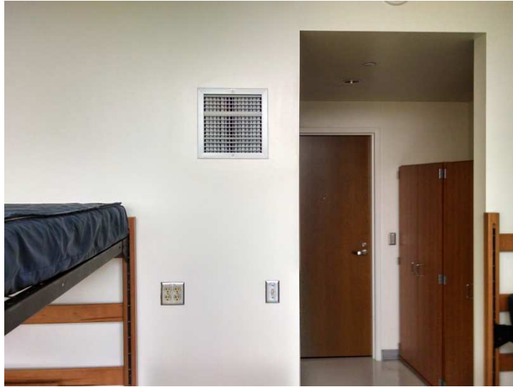
Return grill in each room connects to ventilation system.
