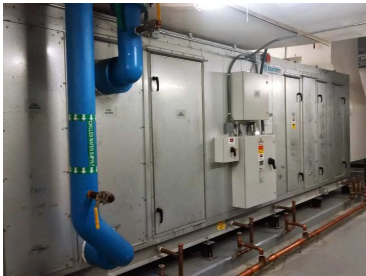
Air handling unit in the penthouse of Summit. Notice the copper condensate drain retroactively added.
