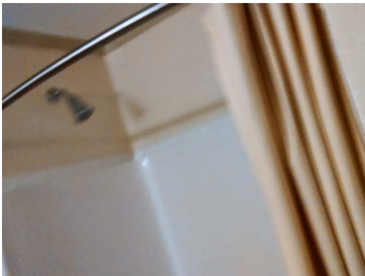
Curved shower rods in the Mountaineer baths have caused water to leak on the floor in some units.
