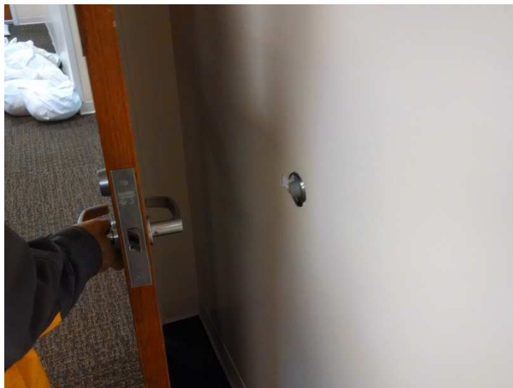
Hole in in a wall at Mountaineer because the door stop does not have adequate blocking behind it.
