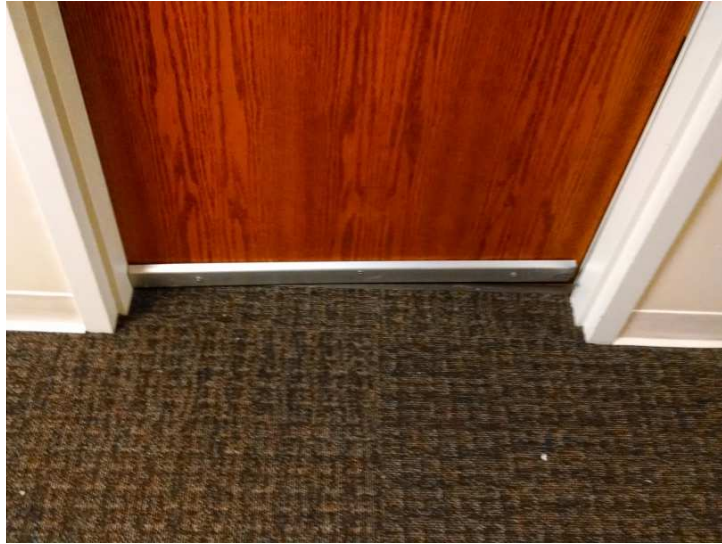
Smoke seals at the threshold of each door have been removed so the doors can completely close.
