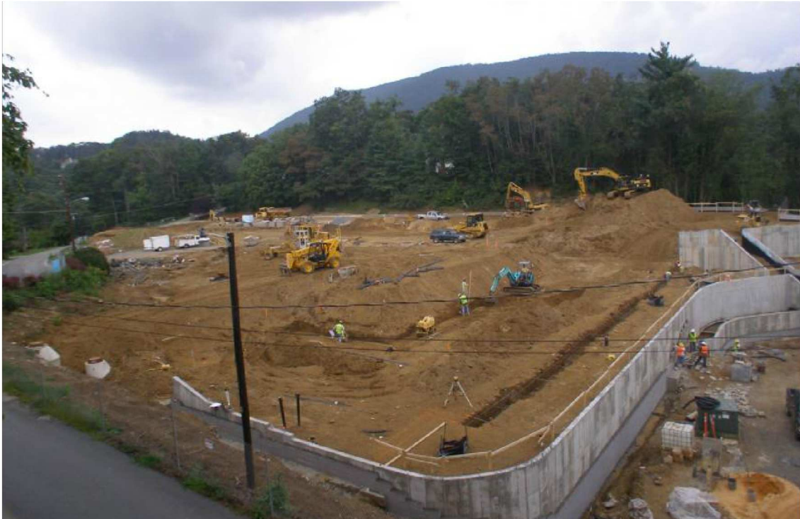
Figure 34. Mountaineer Hall during construction on August 24 th , 2010. Some footings have been dug, and reinforcing steel placed, while others are currently being dug (Hunter-Saak, 2014. Reprinted with permission).
