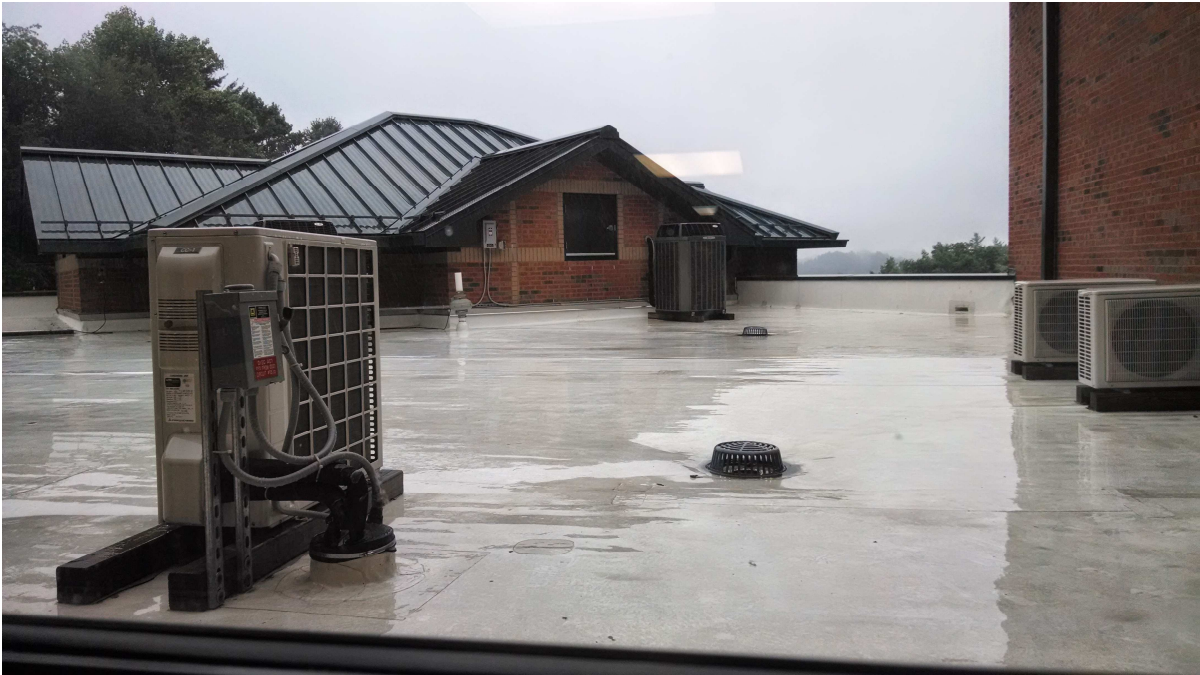
Figure 44. Condensing units of split-system heat pumps visible on the roof of Mountaineer Hall. Also visible near the attic access door is one of the 42 radon mitigation fans (photo by author).
