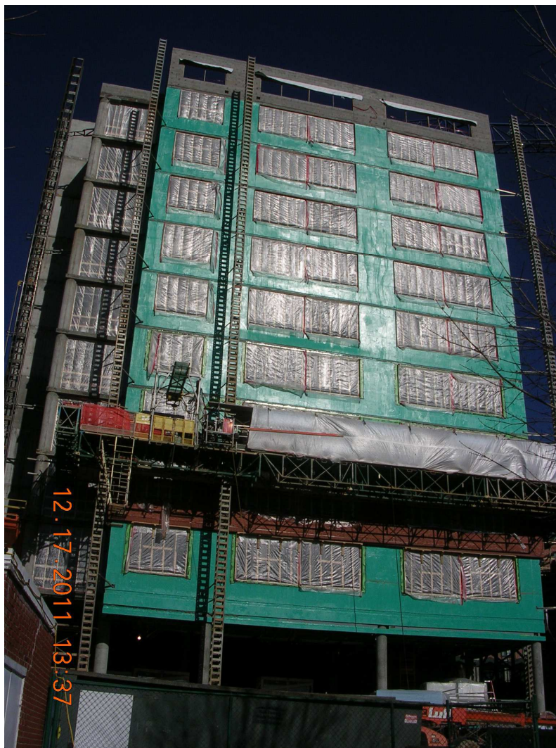
Figure 37. Temporary windows and walls constructed of wood and polyethylene sheeting during the construction of Summit Hall (photo courtesy of John Schlobohm).
