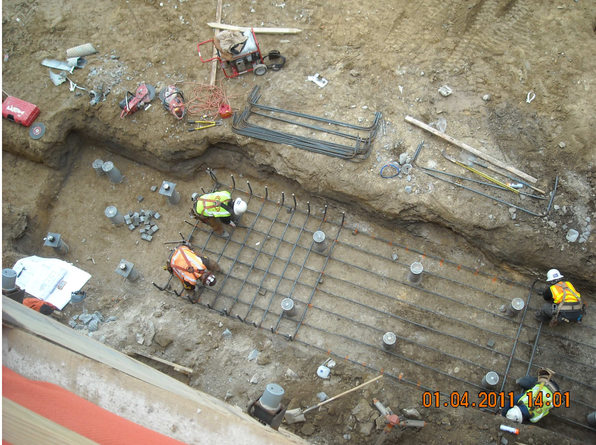
Figure 45. Deep foundation piles are installed, and reinforcing steel is being tied for pile caps on the foundation of Summit Hall. Notice the date of January 2011. Although construction started in Summer of 2010, building construction was just ramping up in 2011 (photo courtesy of John Schlobohm).
