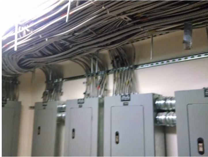
Closer look at the web of MC cables powering Mountaineer.
