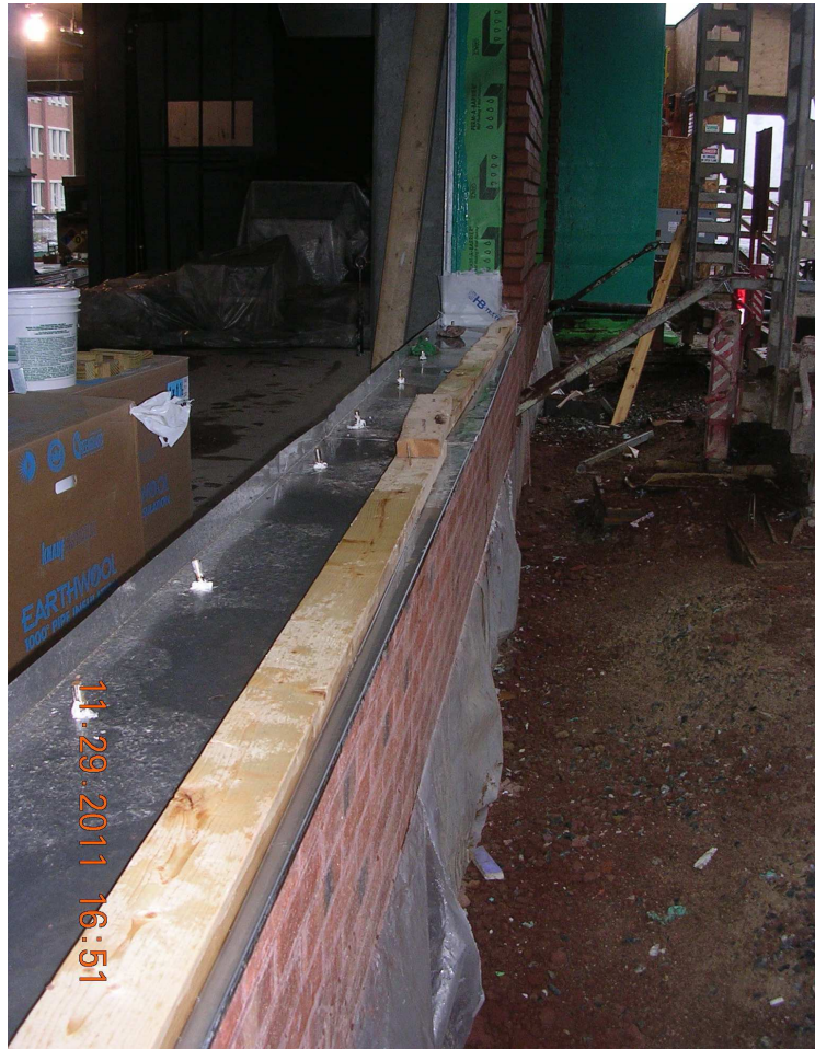
Figure 38. Sheet metal flashing installed under pre-cast concrete window sills. Notice the steel studs protruding through the flashing that caused the windows to leak after occupancy (photo courtesy of John Schlobohm).
