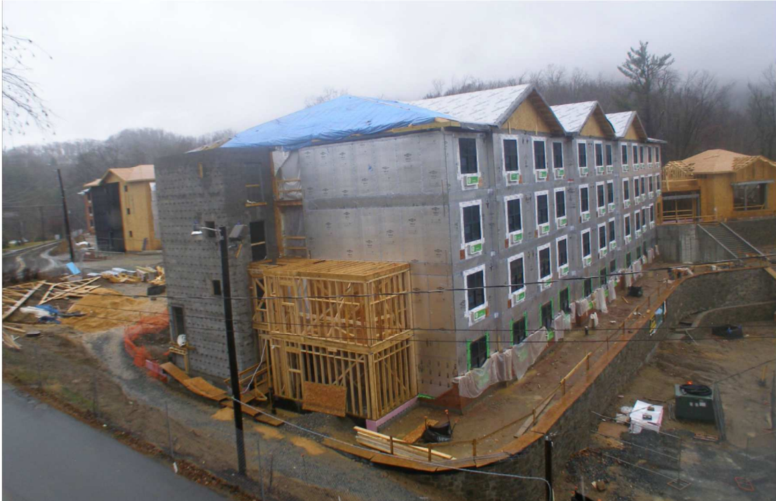
Figure 33. Mountaineer Hall during construction on November 30 th , 2010. All modules are set and brick is being laid on the first floor (Hunter-Saak, 2014. Reprinted with permission).
