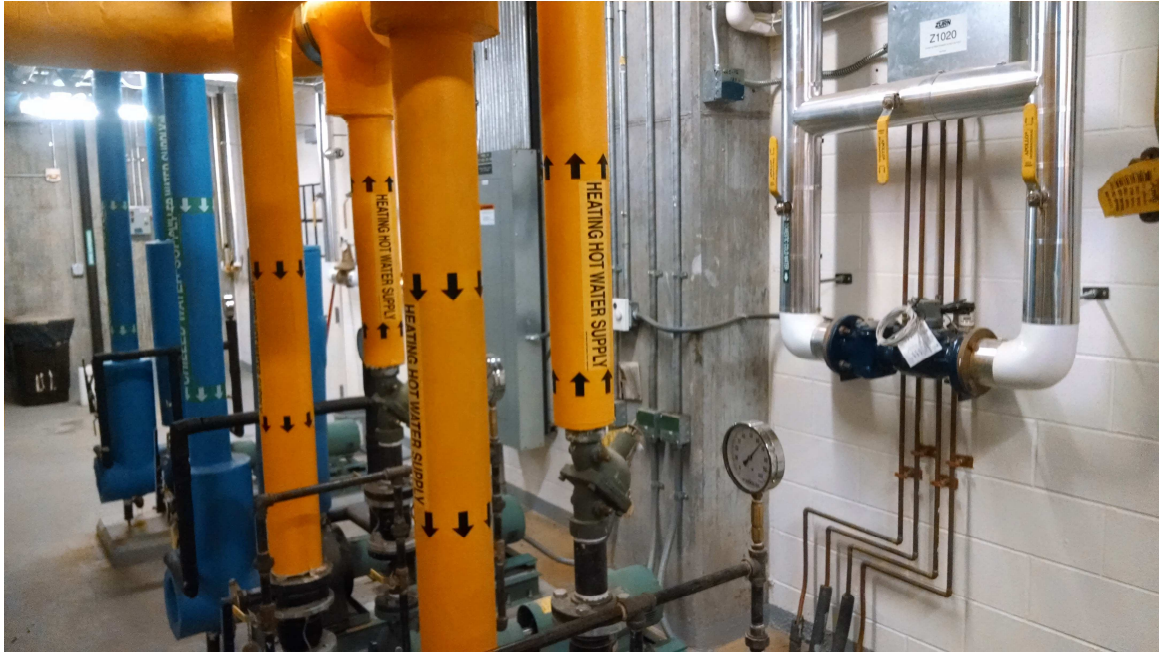
Figure 43. One basement mechanical room of Summit Hall with chilled water and building hot water lines connected to circulation pumps (photo by author).
