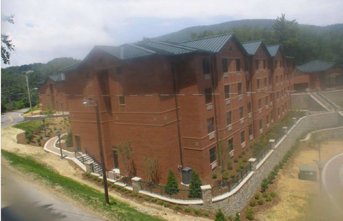
Figure 35. Mountaineer Hall during construction on June 13 th , 2011. The building is complete (Hunter-Saak, 2014. Reprinted with permission).
