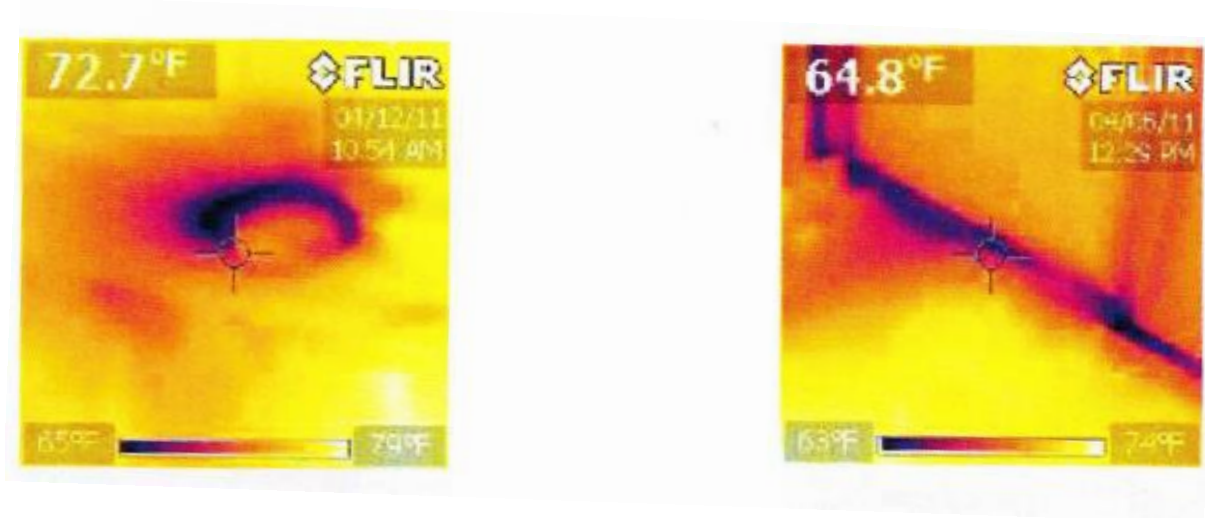
Figure 7. Infiltration around recessed light and attic access door.
