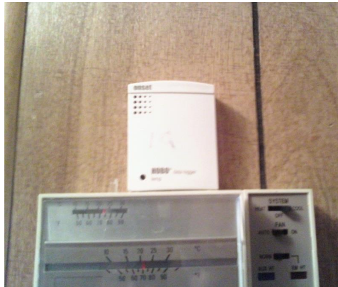
(c) Zone temperature sensor placed inside trailer over thermostat.
