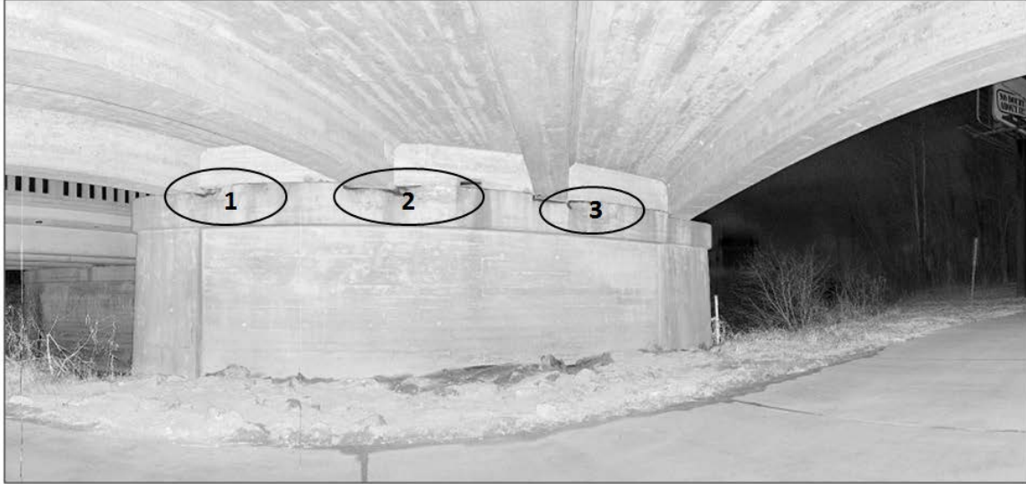
Figure 3.9 LiDAR scan for damage detection in bridge 590147 (Charlotte, NC)
