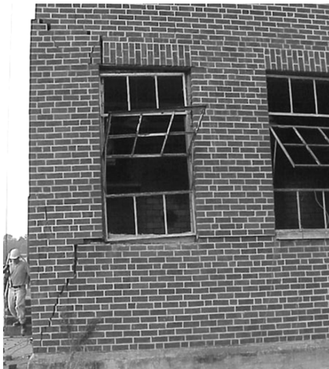
FIGURE 7.26: Photo of damage observed at the intersection of Walls #2 and #3.
