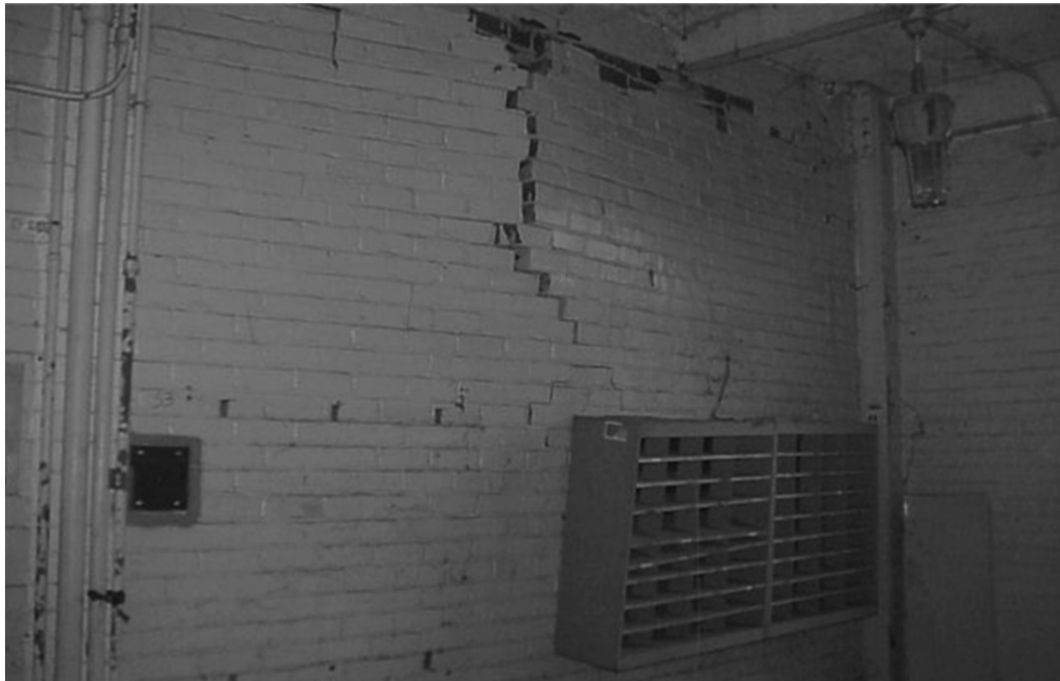
FIGURE 7.22: Photo of damage observed in Wall #1.
