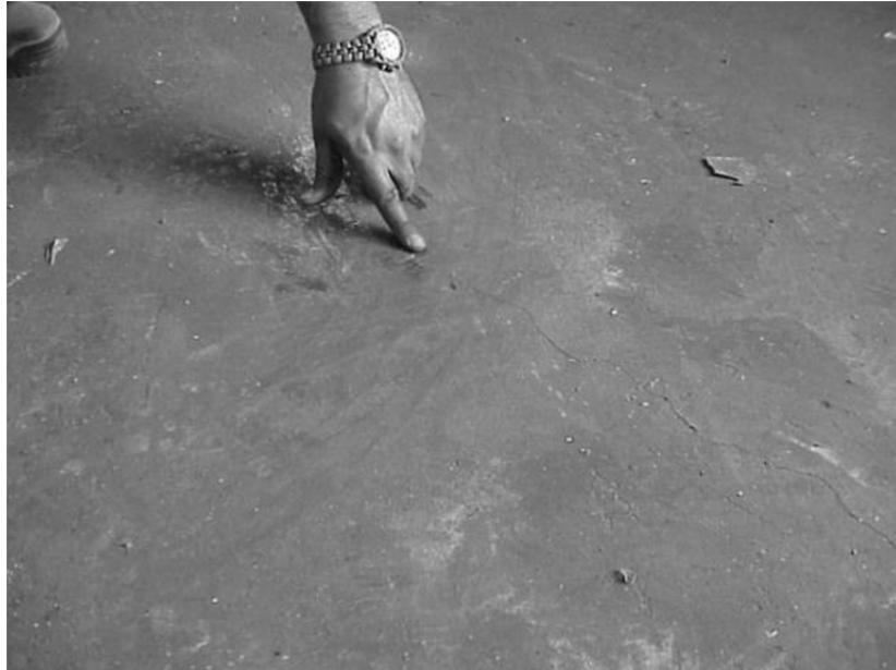
FIGURE 2.12: Crack on top surface of A1 blast chamber ceiling directly above charge location. Crack aligned with embedded I-shaped member supporting the slab.
