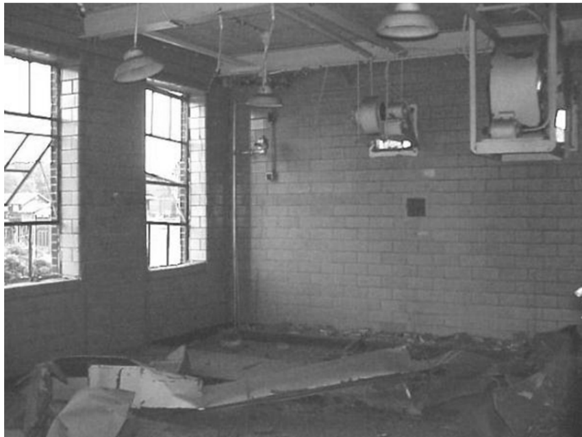
FIGURE 2.15: Post-test view of the location B blast chamber showing extensive damage to nonstructural items.
