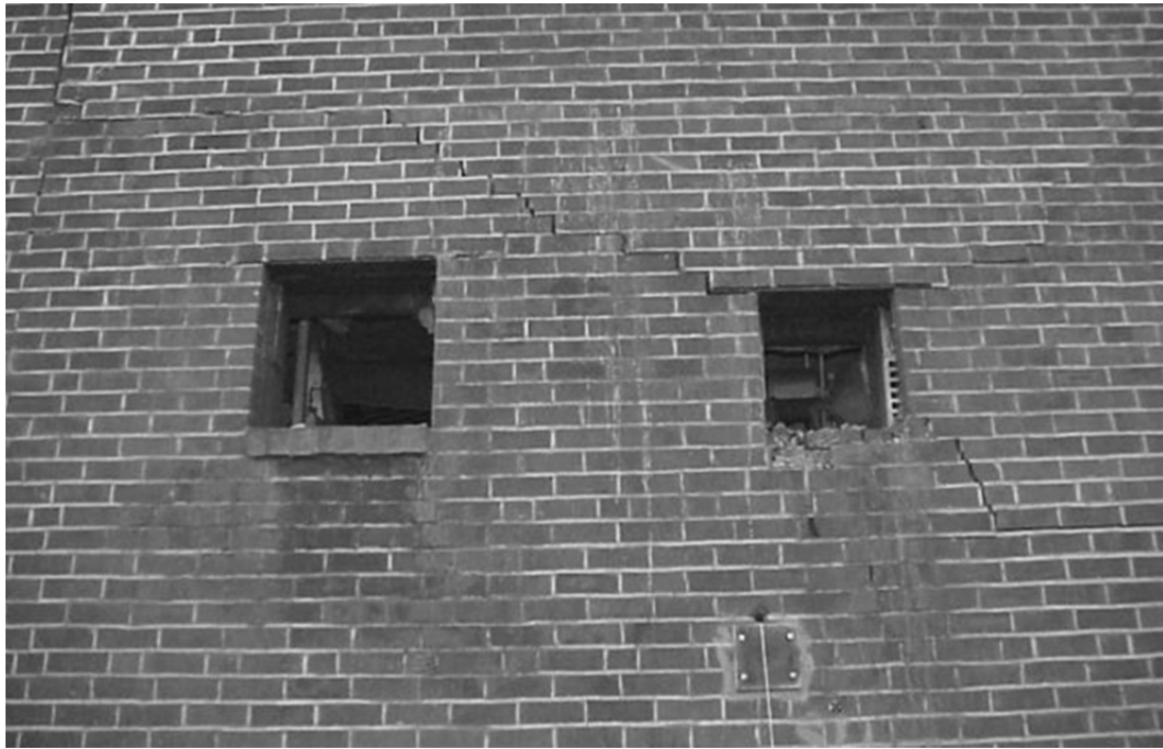
FIGURE 7.24: Photo of damage observed in Wall #2 near mid-panel.
