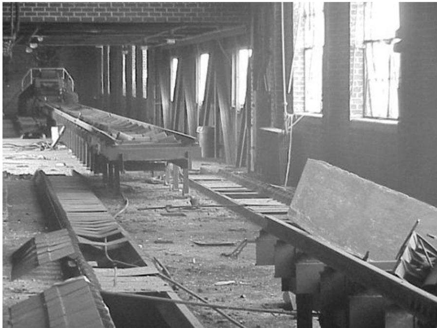
FIGURE 2.13: Post-test view of A2 blast chamber showing damage to non-structural components. Note the bent steel plates at lower left.
