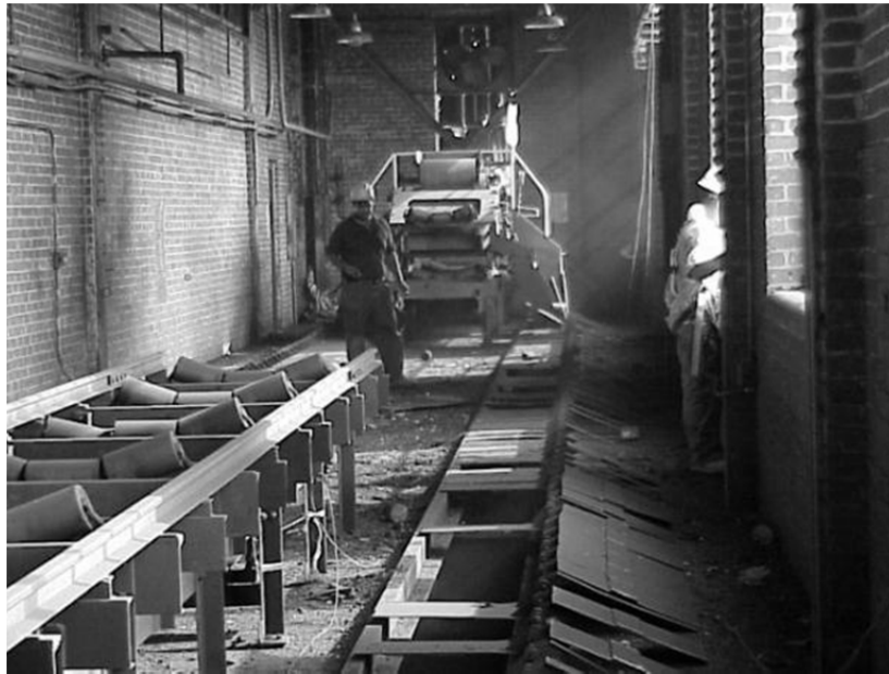
FIGURE 2.11: Post-test view of A1 blast chamber showing little to no structural damage.
