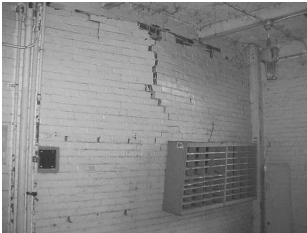
FIGURE 2.16: Post-test view of Wall #1 from outside the blast chamber showing heavily damaged infill panel.
